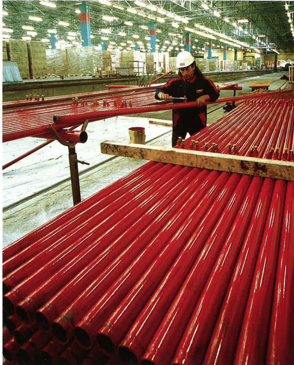
▼ Tunzini Protection Incendie put in the fire protection system at Seita's plant in Riom (Puy-de-Dôme), installing sprinklers throughout the building.
