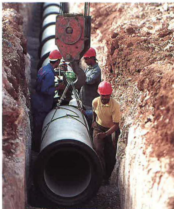
Reinforcement work on the water main north of Agadir (Morocco) carrying water from the Dkhila dam.
