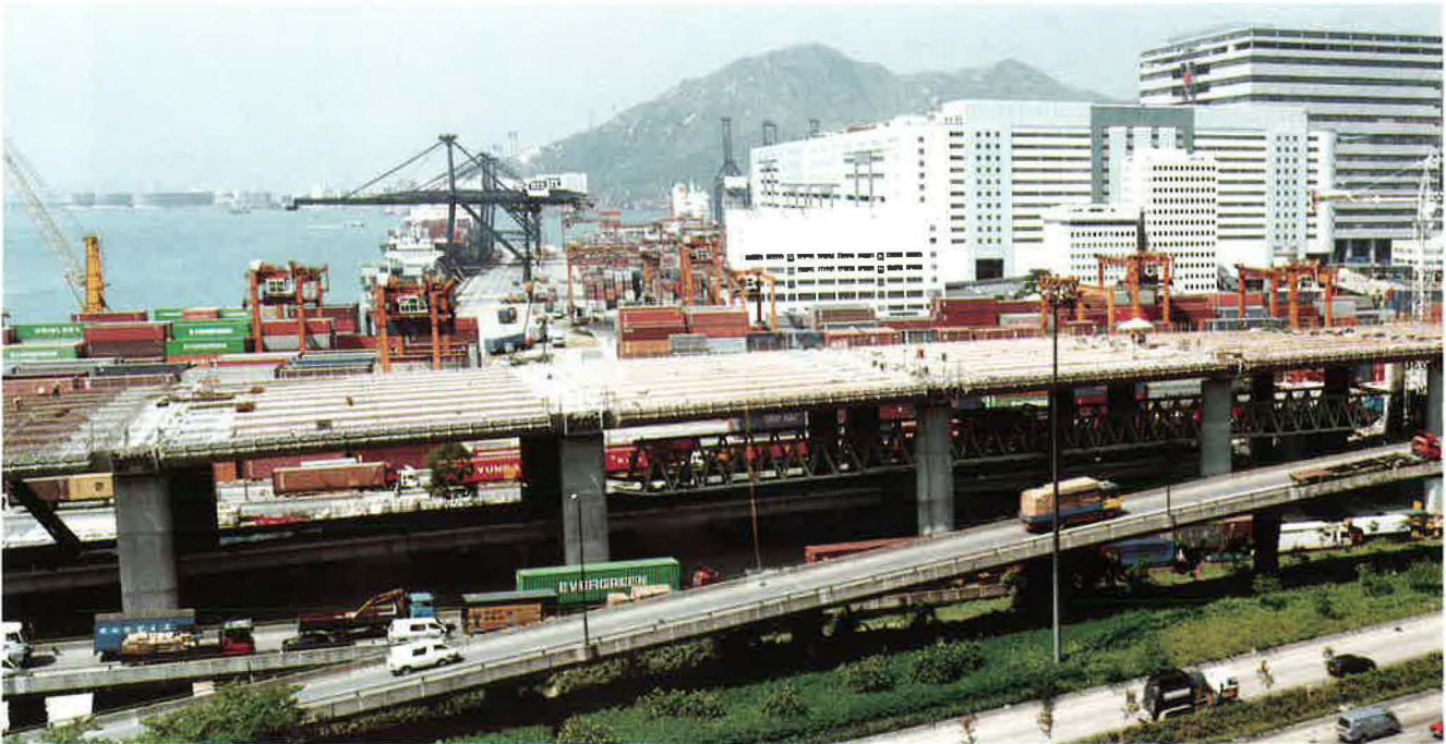
The Kwai Chung viaduct is a key link in the infrastructure program for the new Hong Kong airport. 3.5 km long, with a total deck surface three times that of the Normandy bridge, this viaduct is being built in a dense urban setting, on top of several busy road and rail arteries.
