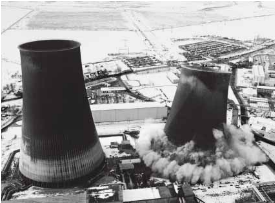
Demolition of one of the cooling towers of the Lippendorf power station near Leipzig in Germany.
