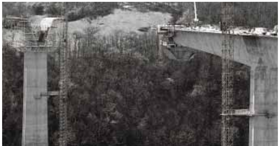
The Tanus viaduct , carrying the RN88 over the Viaur, has set a new record - a central pier 130 metres in height and a deck spanning 190 metres.
