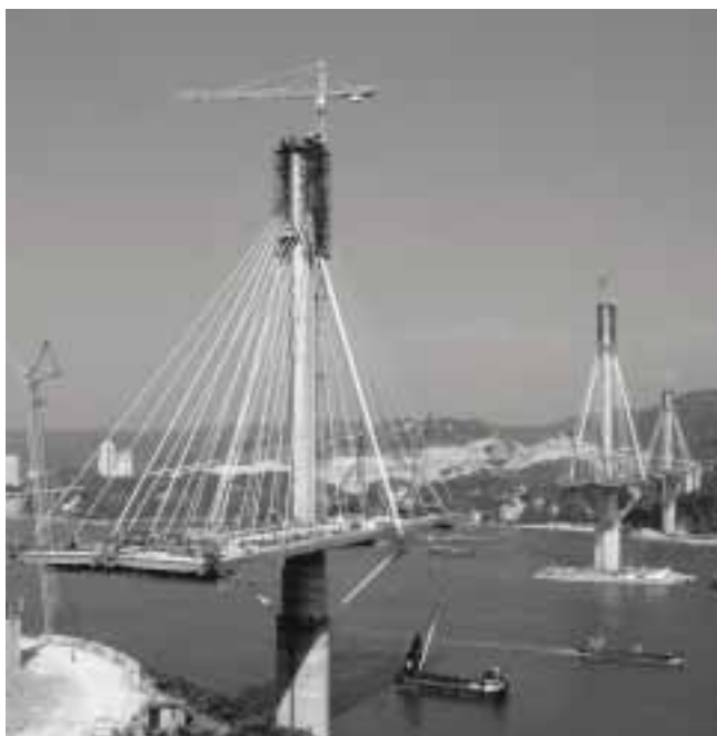
The Ting Kau cable-stay bridge in Hong Kong comprises three pylons respectively 167, 194 and 162 metres in height, and two central spans 475 and 448 metres long.
