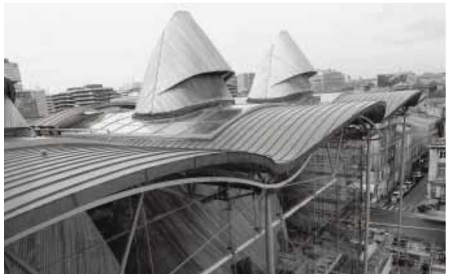
In the new Bordeaux courthouse Tunzini installed the air-conditioning system. The complex comprises five office levels and seven court rooms (architect: RRogers).
