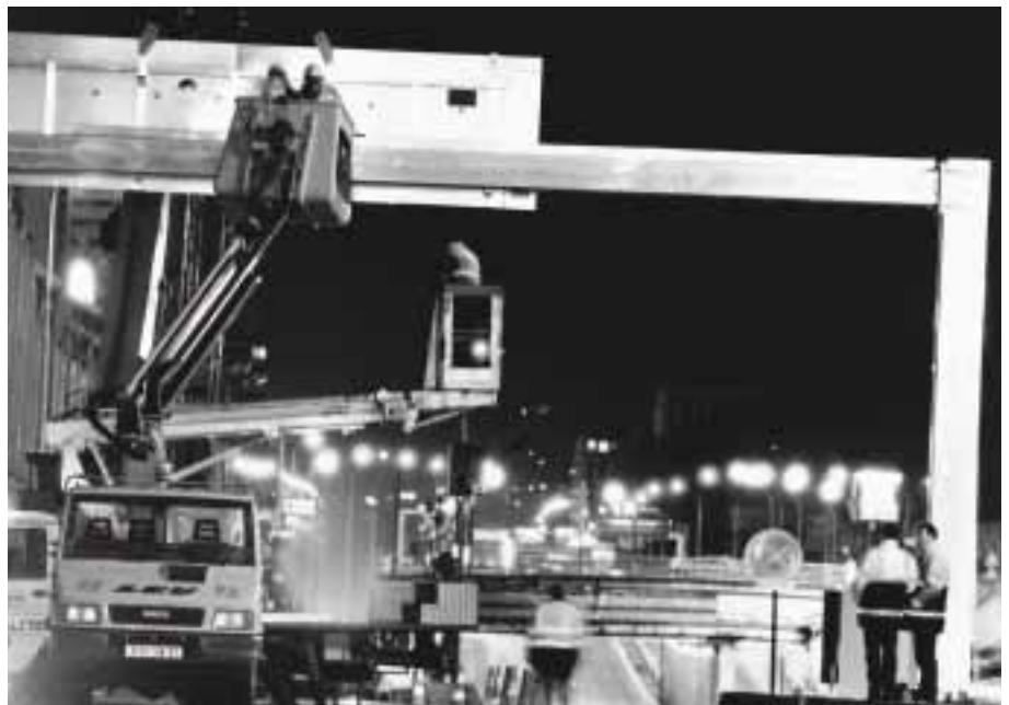
Installing electronic information board, video surveillance systems, and replacing transmission cables on the Paris ring-road.
