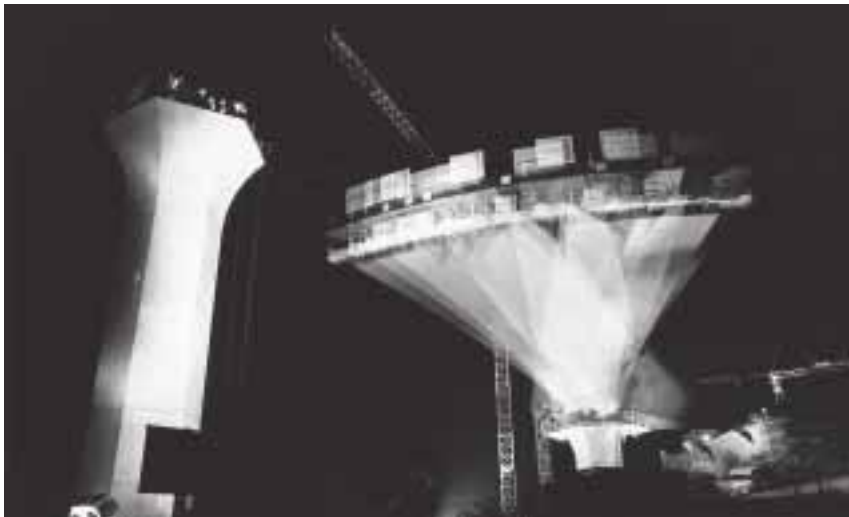
The Ventabren viaduct that will carry the Mediterranean TGV line : the second beam, that was pre-fabricated parallel to the motorway without disrupting traffic, is rotated through 30°.
