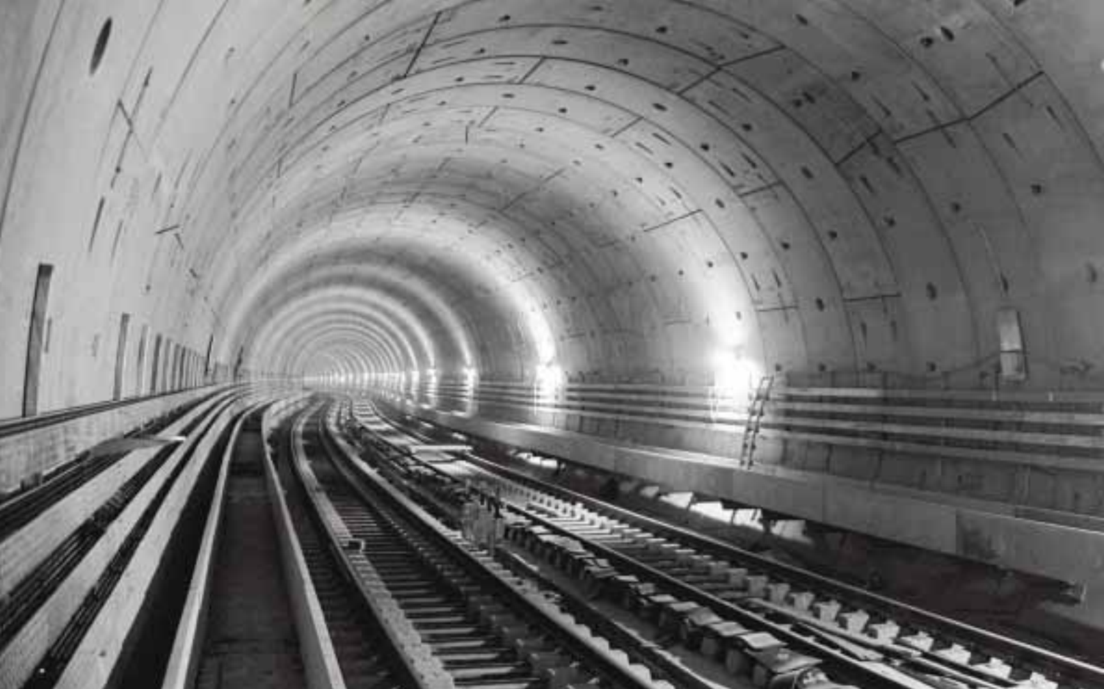
Line 2 of the Cairo underground is being extended towards Gizeh. The last section of the tunnel was bored under the two arms of the Nile.
