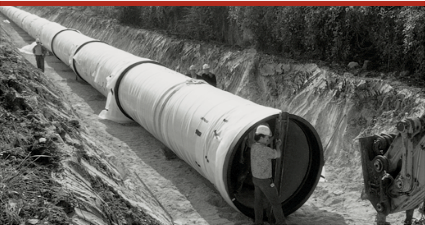
Some 250 metres of 1,800mm diameter cast iron pipe being installed as part of the Avre aqueduct in Auteuil-le-Roi, near Paris.
