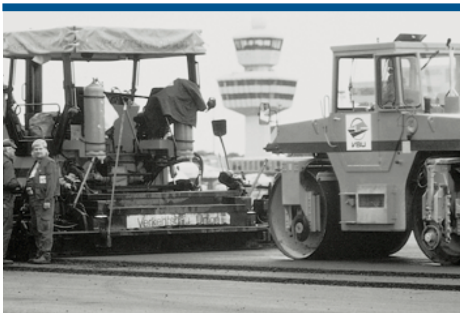
Renovation of the south runway at Berlin's Tegel airport, where 4,000 aircraft take off and land every day.
