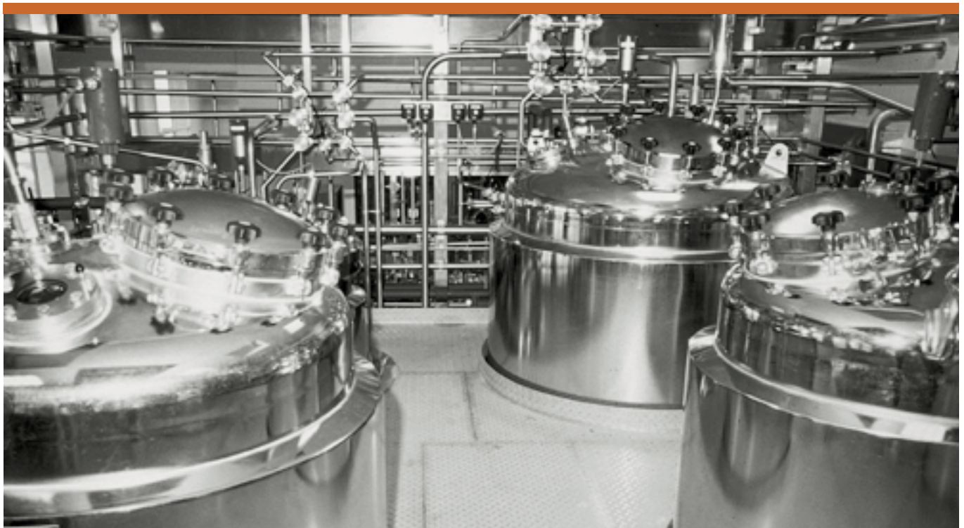
Engineering, electrical installation and instrumentation in the Boehringer pharmaceuticals laboratory at Prenzb erg in Bavaria.
