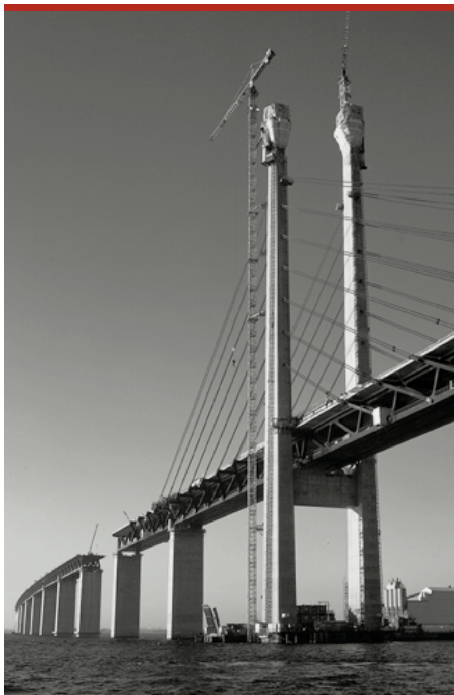
The 16 kilometre Øresund, link between Sweden and Denmark will come into service in 2000.
