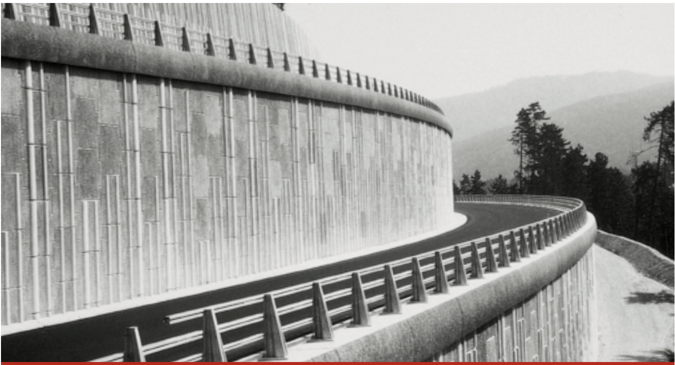
Earth retaining walls are often used to support roads on inclined terrain, as seen here on the A43 motorway near Saint-Michel de Maurienne.
