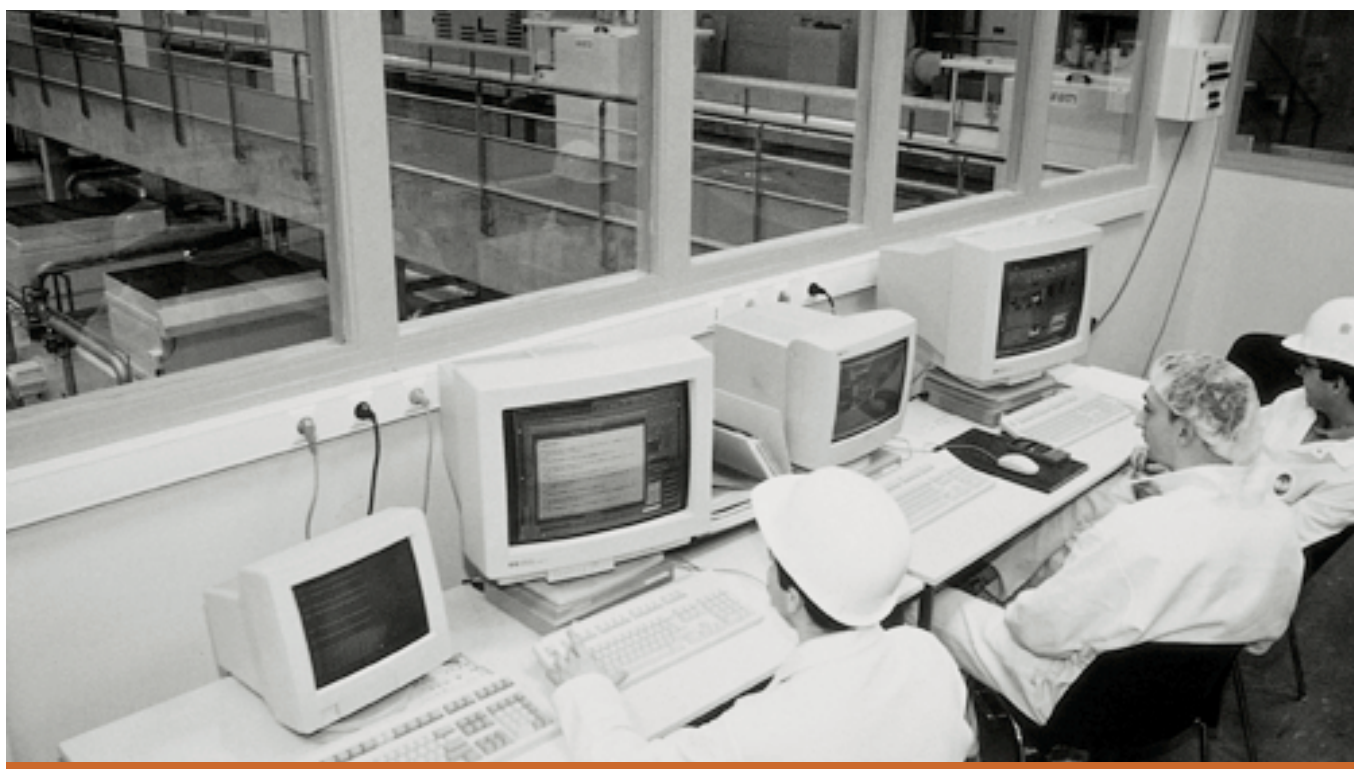
GTIE installed all the electrical engineering, automatic control and monitoring systems in the OGC Cacao cocoa bean processing plant near Rouen.
