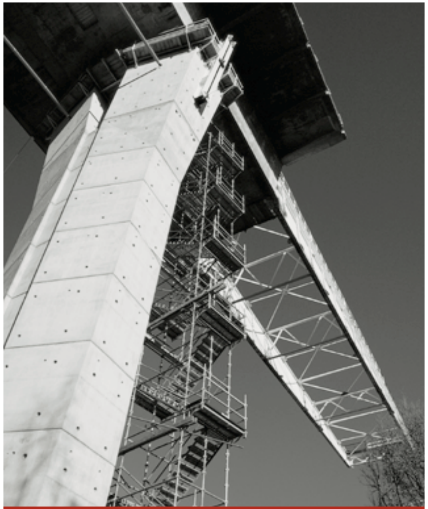
The 280 metre long Bergères viaduct, whose highest pier rises 31 metres, will be part of the A89 motorway that will link Bordeaux to Clermont-Ferrand as of 1999.
