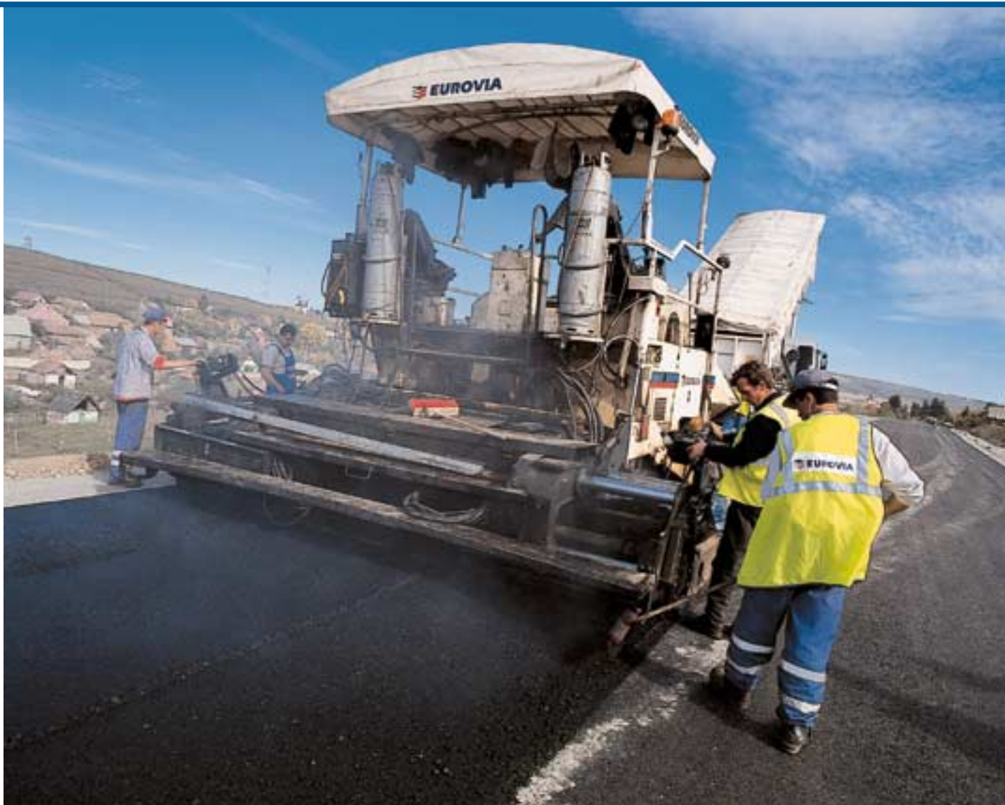
The Brasov to Bogata Hill road rehabilitation project in Romania involved widening 36 kilometres of the RN13 highway.
