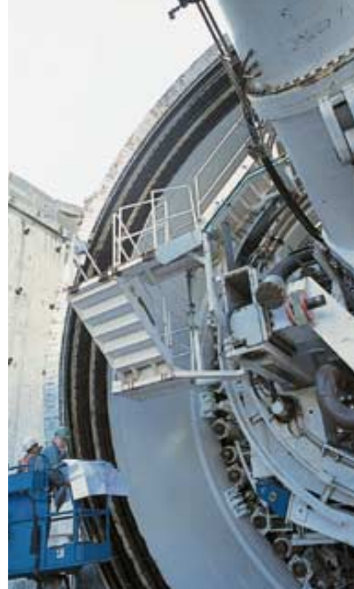
Tunnel-boring operations with a TBM have started on the A86 motorway around the west of Paris. The first toll-paying section will be opened to the public in November 2004.
