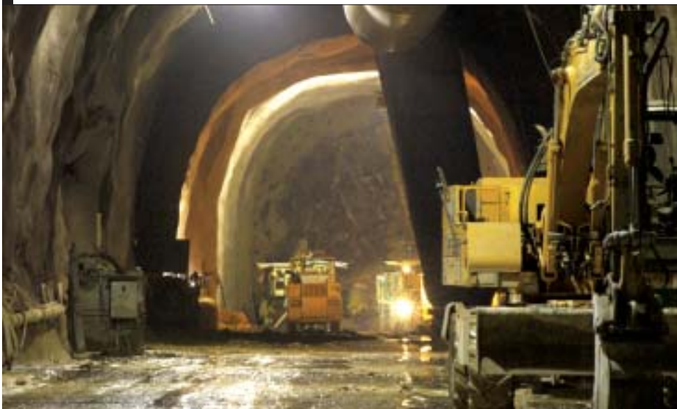
Digging the 6 km Soumagnes tunnel in Belgium, on the Brussels-Cologne high-speed train link
