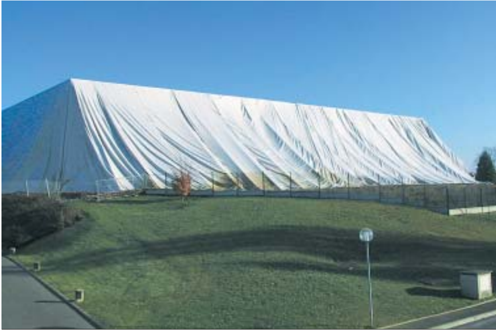
Delair-Navarra developed a near-confinement process that reduces the environmental impact of building demolition ■
