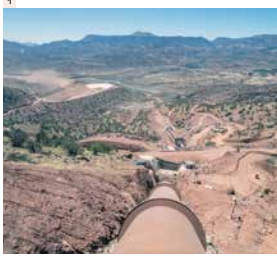
1 Civil engineering works at the Abdelmoumen pumped storage power plant in Morocco.
