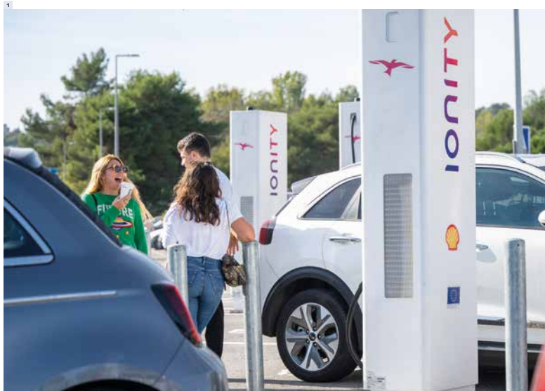
1 A high-power IONITY EV charging station at the Breguières Nord service area (A8) between Nice and Mandelieu in the south of France.
