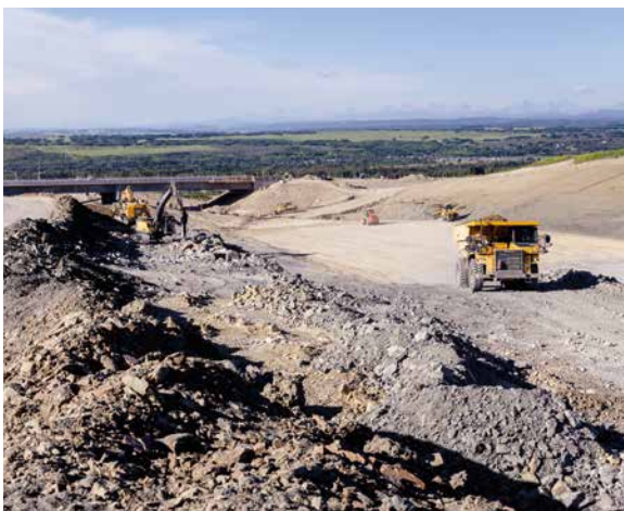
Construction work on the West Calgary Ring Road. This new roadway infrastructure will include four interchanges, seven bridges and a pedestrian underpass.
