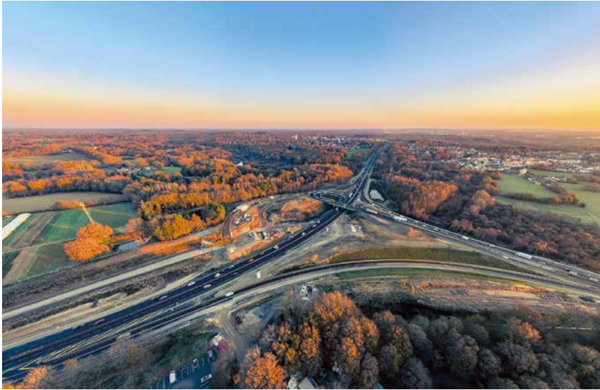
The Porte de Gesvres intersection at the junction between the A11 and the Nantes ring road is being reconfigured as part of the motorway investment plan.
