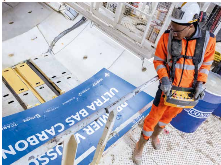
3 Construction of the City Rail Link in Auckland, which will ultimately form a 4 km ring connecting the outer areas to the central business district and link up with the existing transport system.
