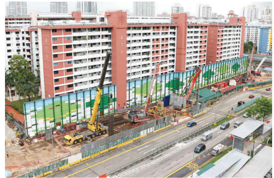
In Singapore, Soletanche Bachy is working on the extension of the Ang Mo Kio metro station, including its six entrances, two microtunnel-bored underpasses, a cut-and-cover tunnel and two TBM-excavated tunnels. This project uses the very latest Hydroraise® (HF8c) developed by Soletanche Bachy.
