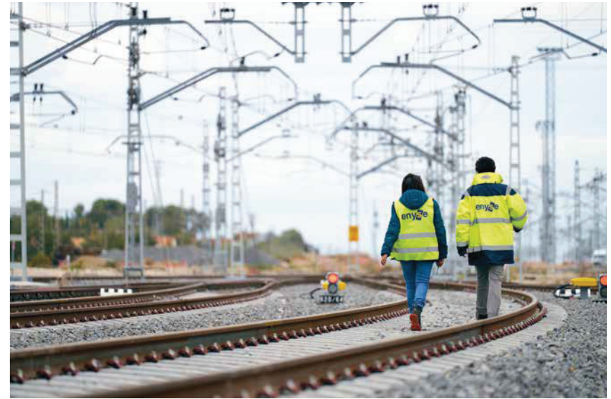
Installation and commissioning of the new electronic interlocking system technology at Vicálvaro intermodal terminal, Madrid (Spain).
