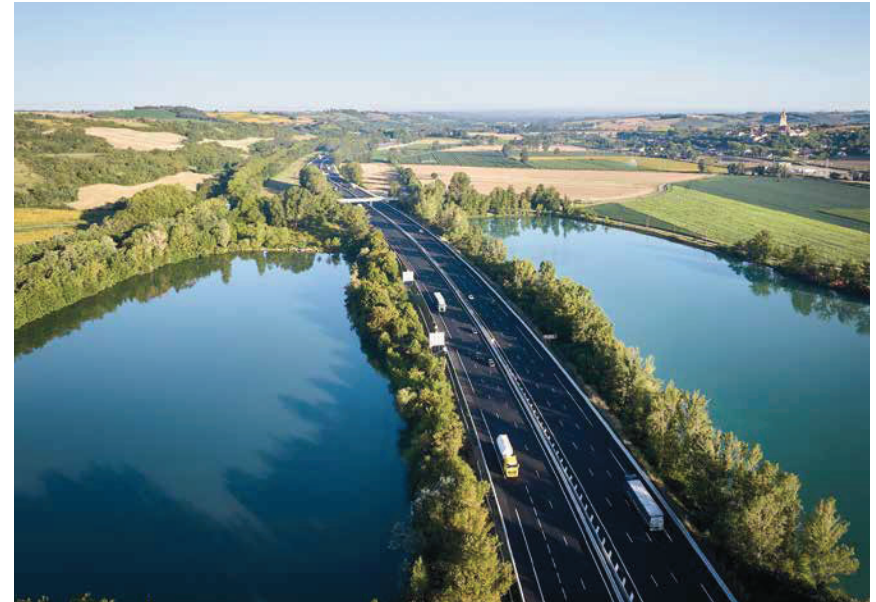
Widening works to create a three-lane dual carriageway on a 35 km stretch of the A61 motorway between Toulouse and Narbonne. Above is a section near the Port-Lauragais service areas.
