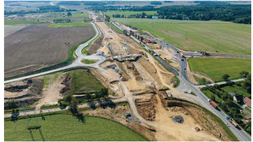
Eurovia CS is working on the construction of the D4 motorway as part of the first motorway public-private partnership in the Czech Republic, with VINCI Highways as the concession company. The new road will enhance the connection between the rural region of South Bohemia and Prague.
