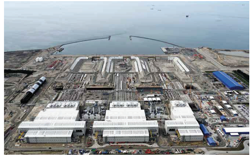
Construction of a precast concrete plant for the 89 sections of the Fehmarnbelt tunnel, the world's longest immersed tunnel, in Denmark was completed in August 2023.
