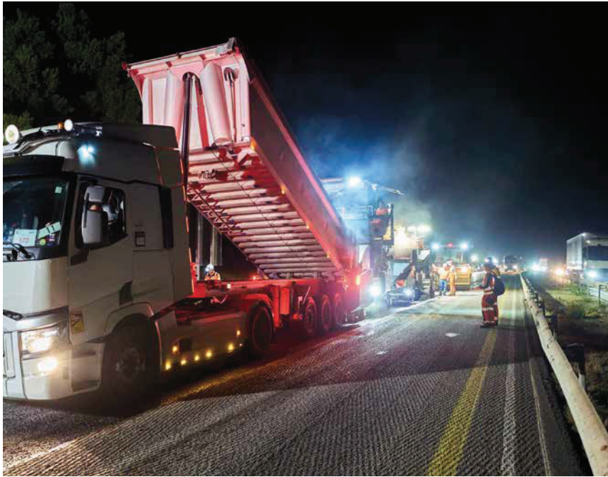
On the A61 resurfacing project between Carcassonne and Lézignan, a significant portion of the asphalt pavement from the old road was reused in the new one.
