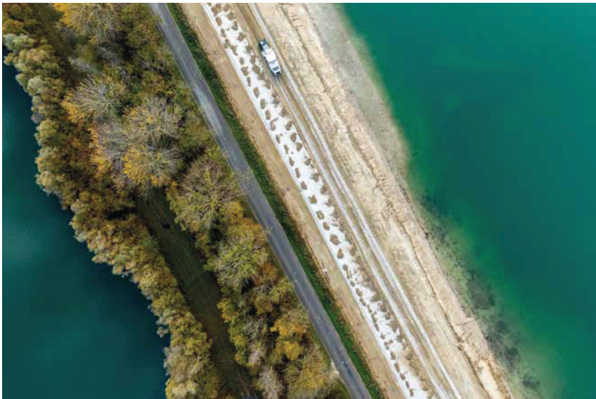
VINCI Construction teams are taking part in the vast La Bassée pilot project at Châtenay-sur-Seine (Seine-et-Marne) to protect the Greater Paris area from the risk of flooding.
