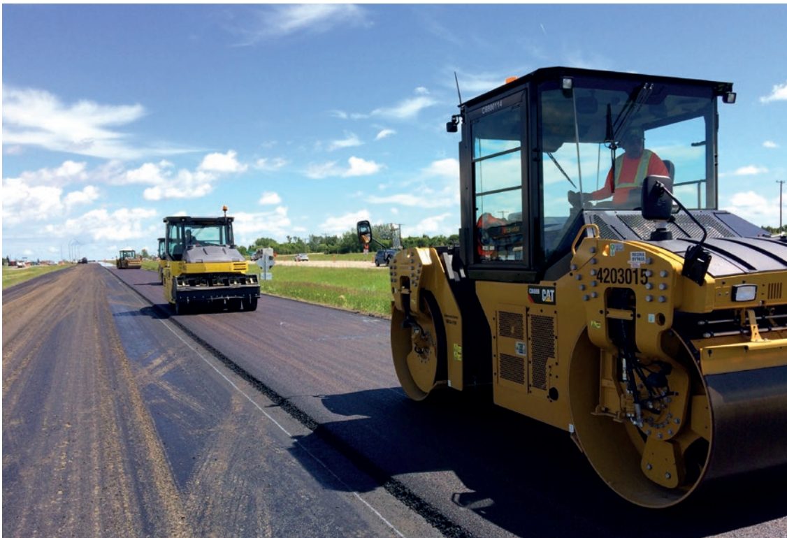
In Canada, construction of the Regina bypass road continues according to the program established.
