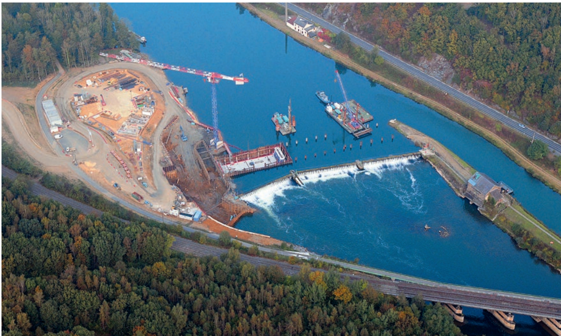
Automation of dams, a key element in the modernization of the French river network.
