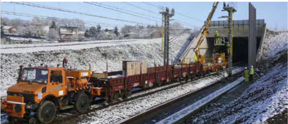
Erecting of catenaries by Engema Rail on the Liège - Cologne high-speed rail route.
