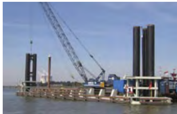
A floating pontoon for river vessels in the middle of the Escaut, at Lillo. Design & Construct: Geka.
