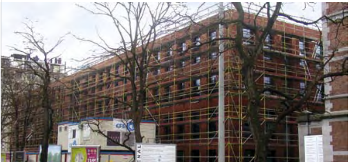
Construction of an office building on the Arsenal site in Brussels. Architect: Archi 2000.
