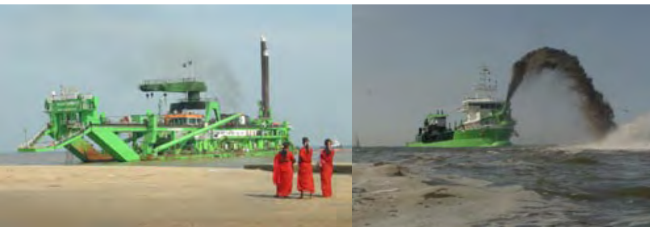
Dredging and reclamation of industrial sites for the extension of the port of Gangavaram in India.
