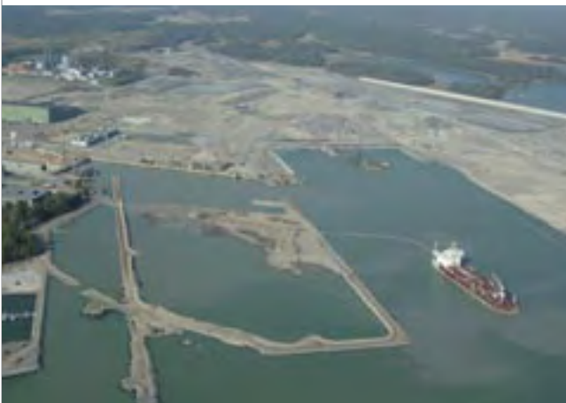
Dredging and reclamation for the extension of Vuosaari harbour, near Helsinki in Finland.
