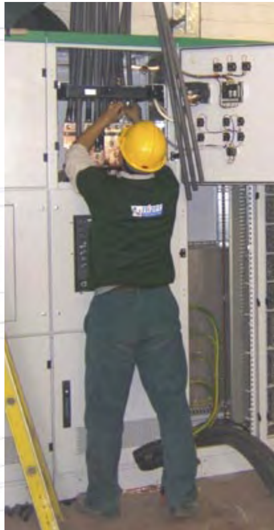
Connecting up instrument panels for the reconitioning of Roselies water-treatment plant. Engineering: IGRETEC.
