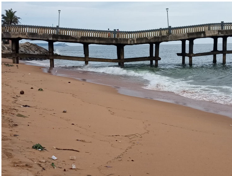
Fig. 5.16. Wide beach gradually got reduced as is seen in Nov 2022 and the Valiyathura pier itself got damaged and became unusable – fair weather beach totally disappeared south of pier while the width of fair-weather beach considerably reduced north of pier
