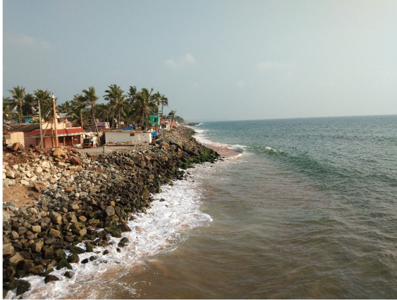
Fig. 5.9b. Higher seawall at Valiyathura after series of repairs and reconstructions for sustaining slumping seawall with no beach on seaward side even during fair season (Photo: fair season 2018),
