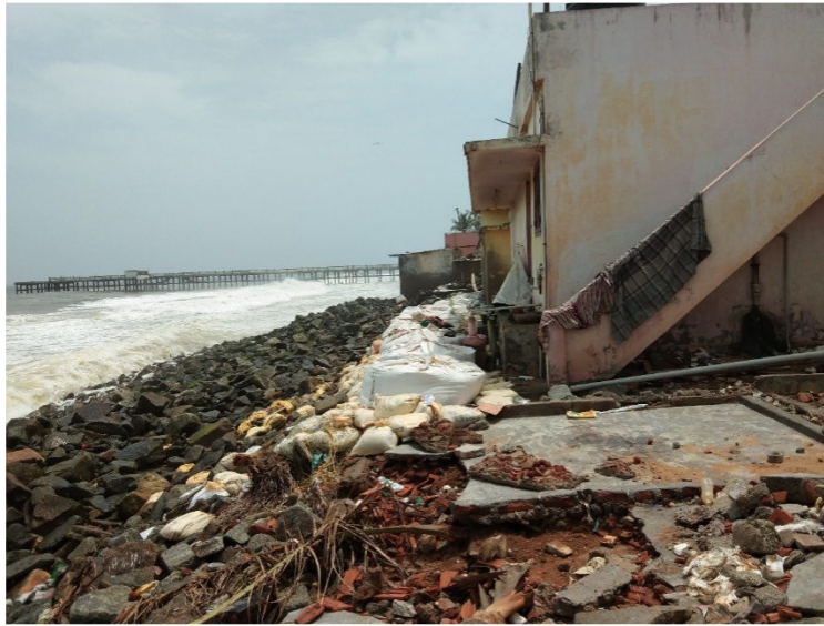
Fig. 5.8. Overtopping waves causing damages to houses – these houses were away from the shoreline, but came close to shoreline when beaches got eroded after seawall construction.
