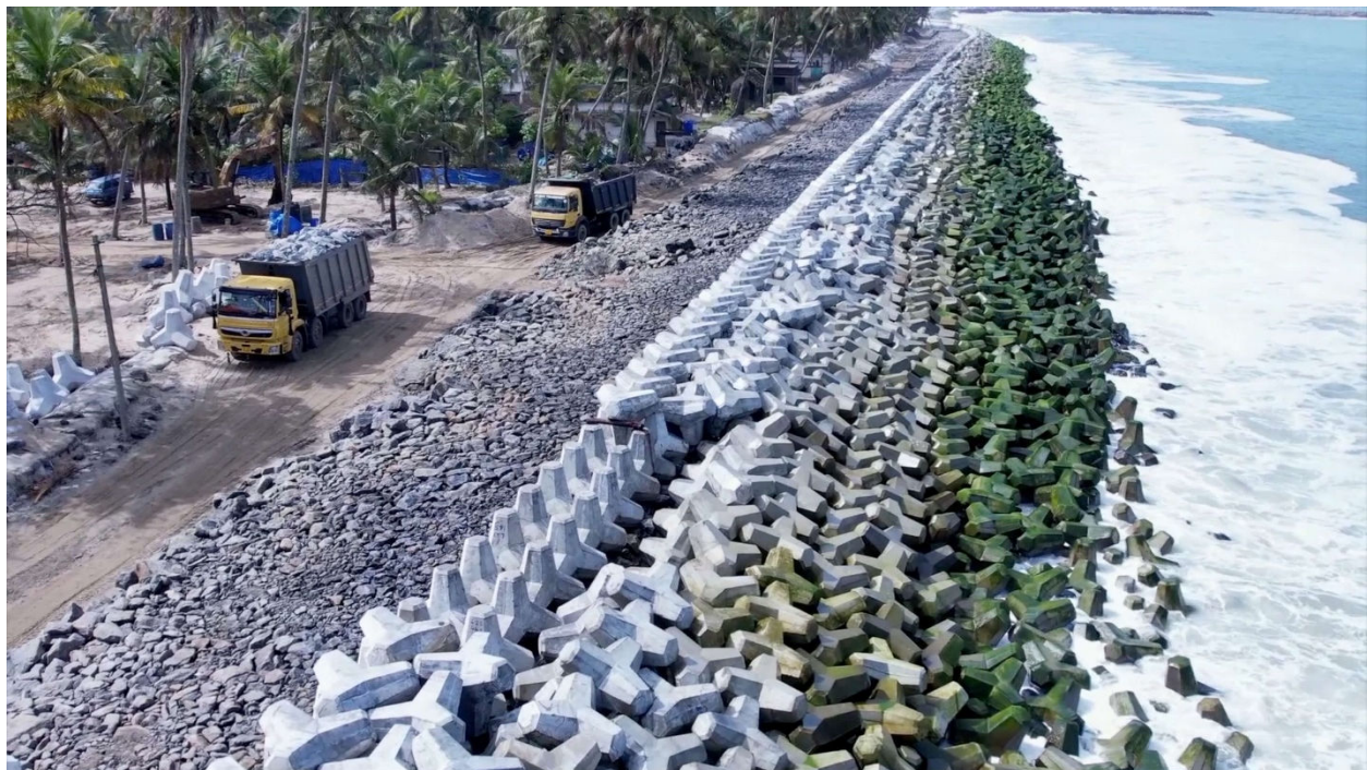
Fig 10.4 The seawall is already being scoured by the waves!
