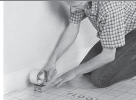
Seal the edge insulation strips using adhesive tape (if a self-levelling screed is to be applied)
