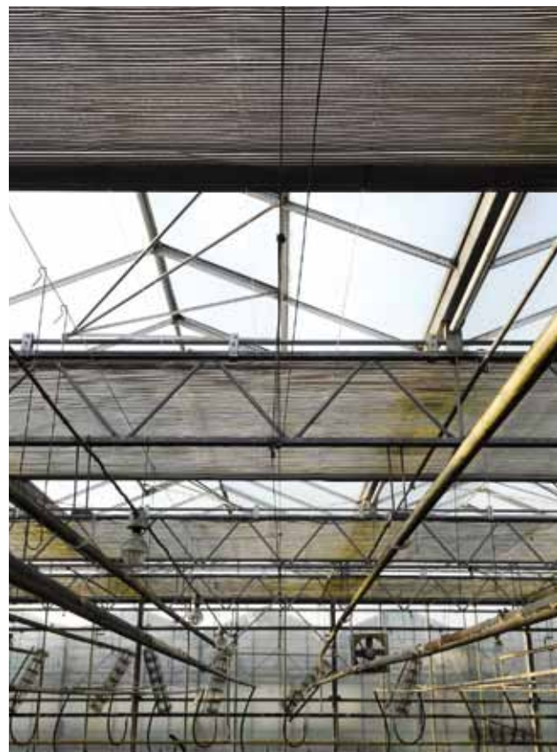
Photo greenhouse shading system
