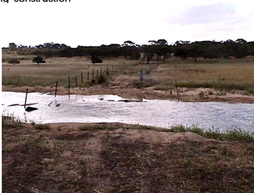
Flood proof fencing on the Dalyup River – note the fence posts are polypipe that will flex during flood events. This section of fencing also has different strainer posts than the fencing along the river, hence won't drag the rest of the fence if impacted by a flood event (photograph Kaylene Parker, WRC).
