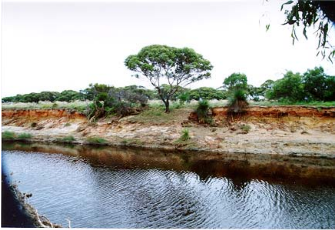
Bank of the Dalyup River showing a channel that is incising and becoming deeper. Note the Yate and how it has retained some of the soil in its root system (photograph Kaylene Parker).
