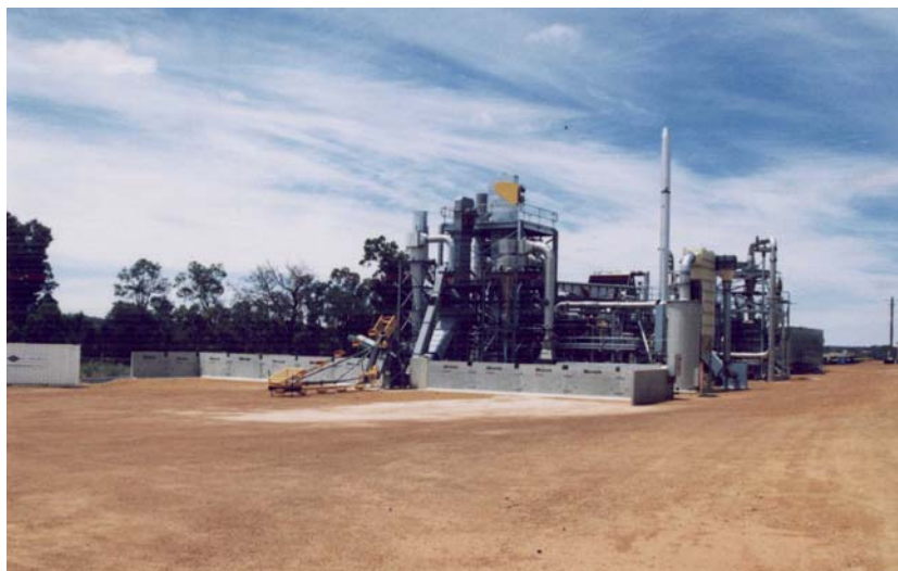
Narrogin IWP plant
