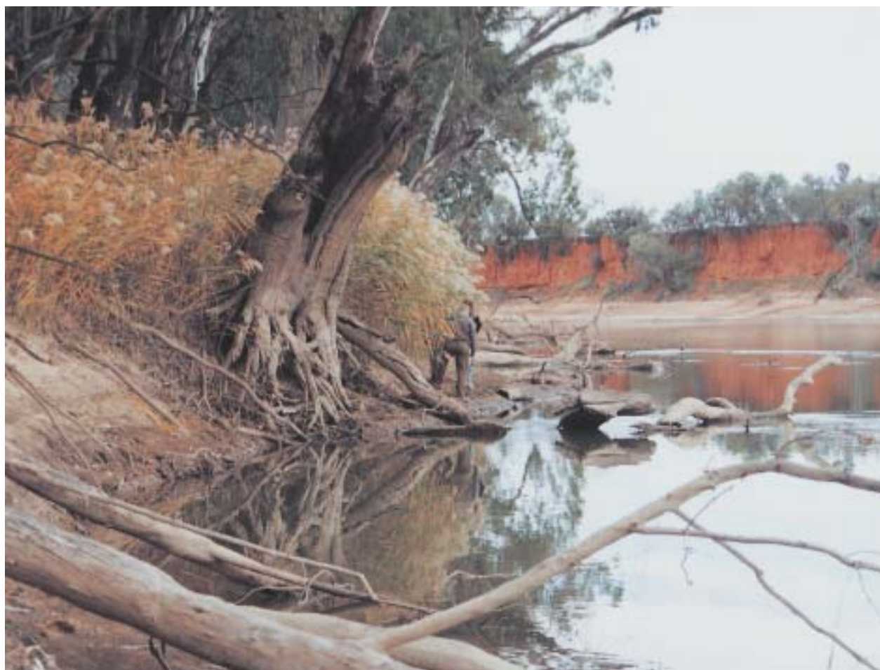
Erosion by scour (left hand side of photo) and mass failure (right hand side) along a large river. Photo Ian Prosser.
