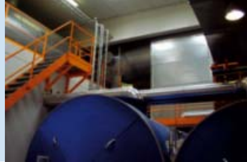
SCR reactor design for the ultra-low emission solution (Grindstedt).
