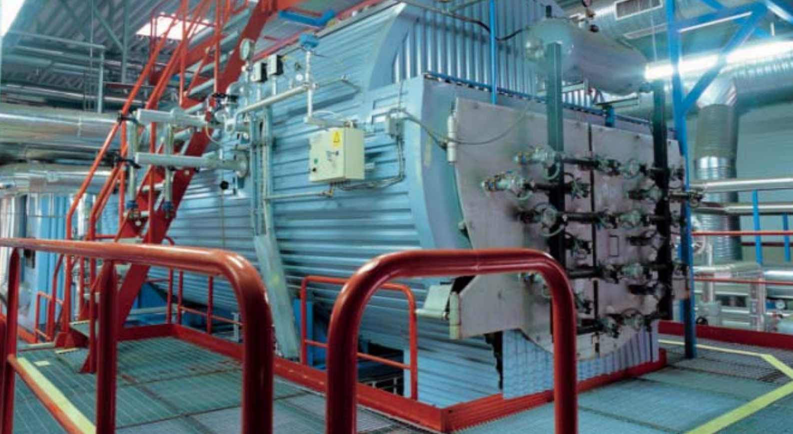
Tranås Energy, Sweden. BioPower, CHP, 15 MW th /1 MW e .
