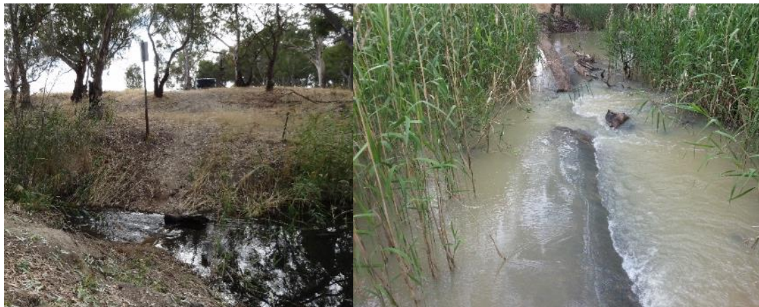
Figure 3-19. Concrete sill on the Wimmera River (left) and Yarriambiack Creek (right) that split all but flood flows between the two waterways.
