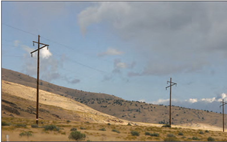
© JERRY LIGUORI FIGURE 4.19: Orientation of power lines parallel to ridges or narrow, low altitude flyways presents a lower risk of collision than perpendicular orientation.
