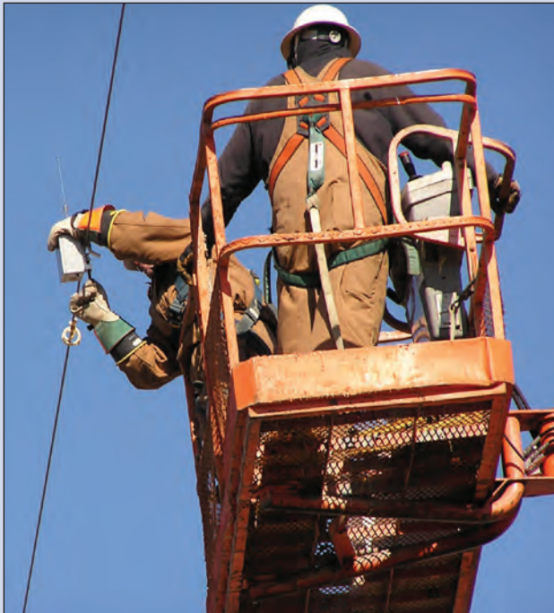
FIGURE 5.2: The Bird Strike Indicator, a tool used to detect bird strikes with power lines, can be installed from a bucket truck or helicopter.
