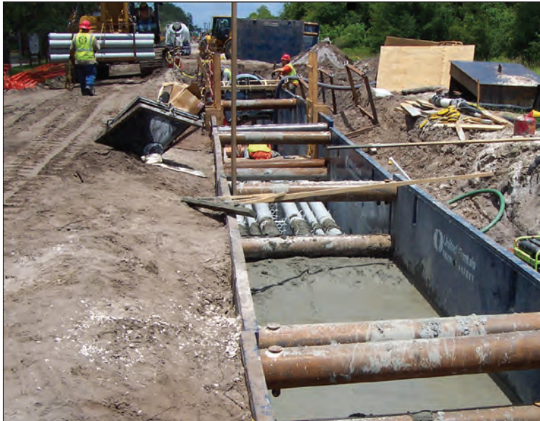
FIGURE 5.6: Buried power lines may be a solution to bird collisions in some instances, but can cost from 3 to 20 times more than overhead lines and have other environmental impacts.
