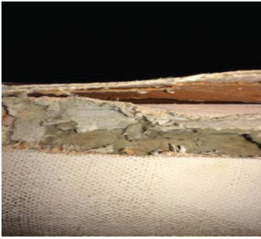
Pipe insulation with multiple layers of non-asbestos paper and 1 layer of ACM
