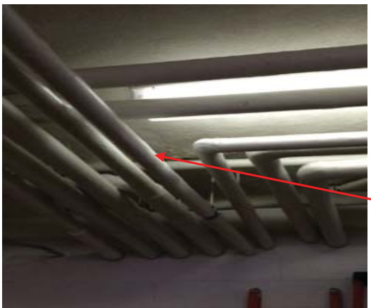
Pipe in Bulk Storage ACM Pipe Insulation (paper with one ACM layer) All fittings (elbows) in photo contain asbestos
