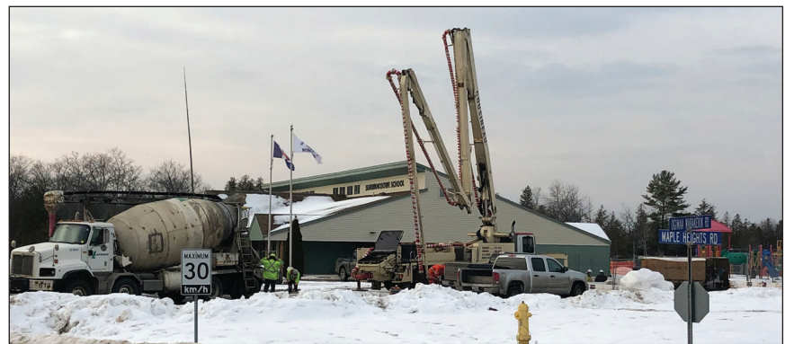
Pouring concrete for the new Maamwe Kendaasing Early Learning and Innovation Centre.
