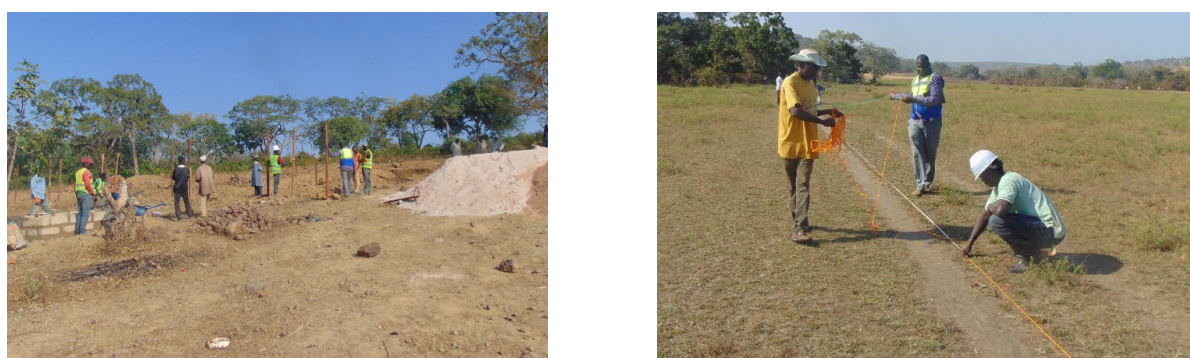
Figure 63. Construction work on Bellakouré market (right); fence-laying work on Lallabara plain (right)
