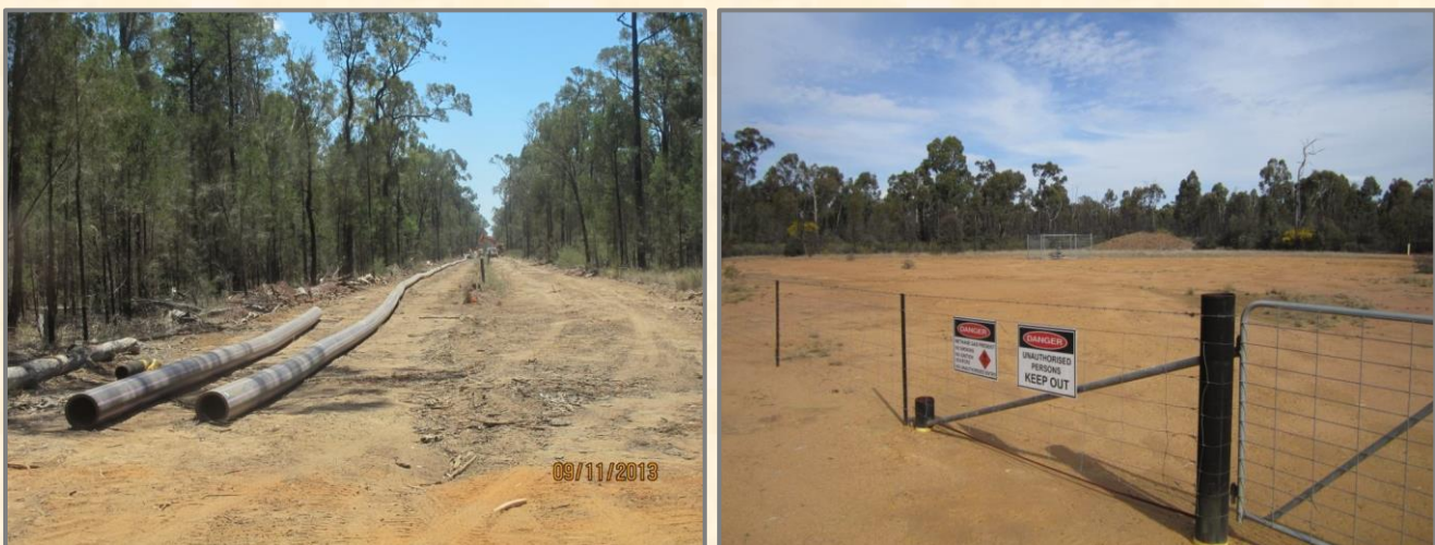
Left: Typical width of pipeline through the forests. Right: Well sites range from 1-2 ha in size.
