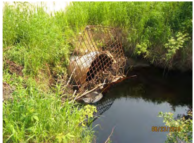
Photo 6. Grate on upstream side of culvert at the water crossing under Grindstone Rd.; effectively blocking fish passage of large bodied fish.
