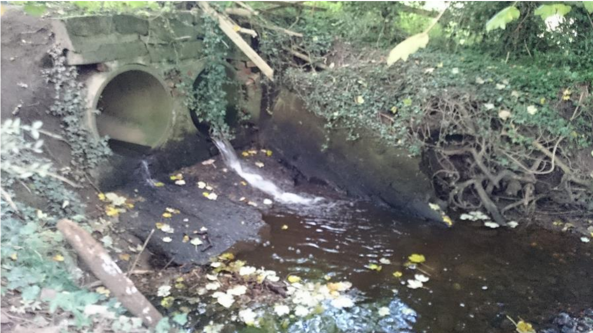
Figure 2. The perched culvert under low flow conditions showing the extent of the degrading sloping apron, and generally poor state of repair of the whole structure. Note the walling on the LB has been undermined by flood waters and is near to collapse.
