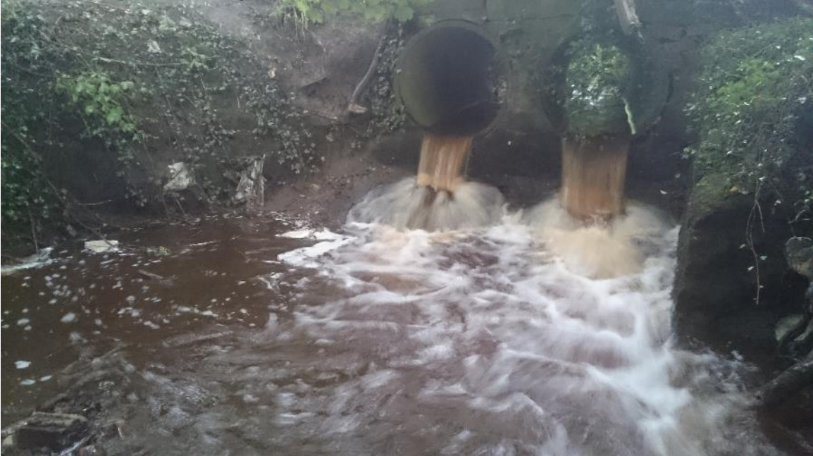
Figure 1. The perched culvert at the mouth of Backstone Beck as it enters the R Wharfe. High flows cascade onto a sloping apron.
