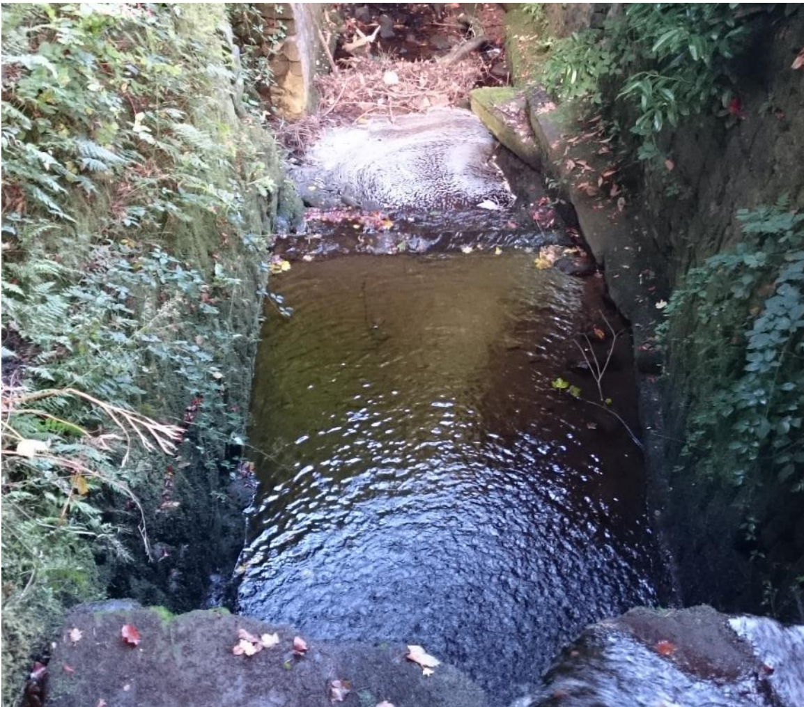
Figure 6. Looking d/s over the walled waterfall, with an estimated headloss of \sim 4\text{m} .
