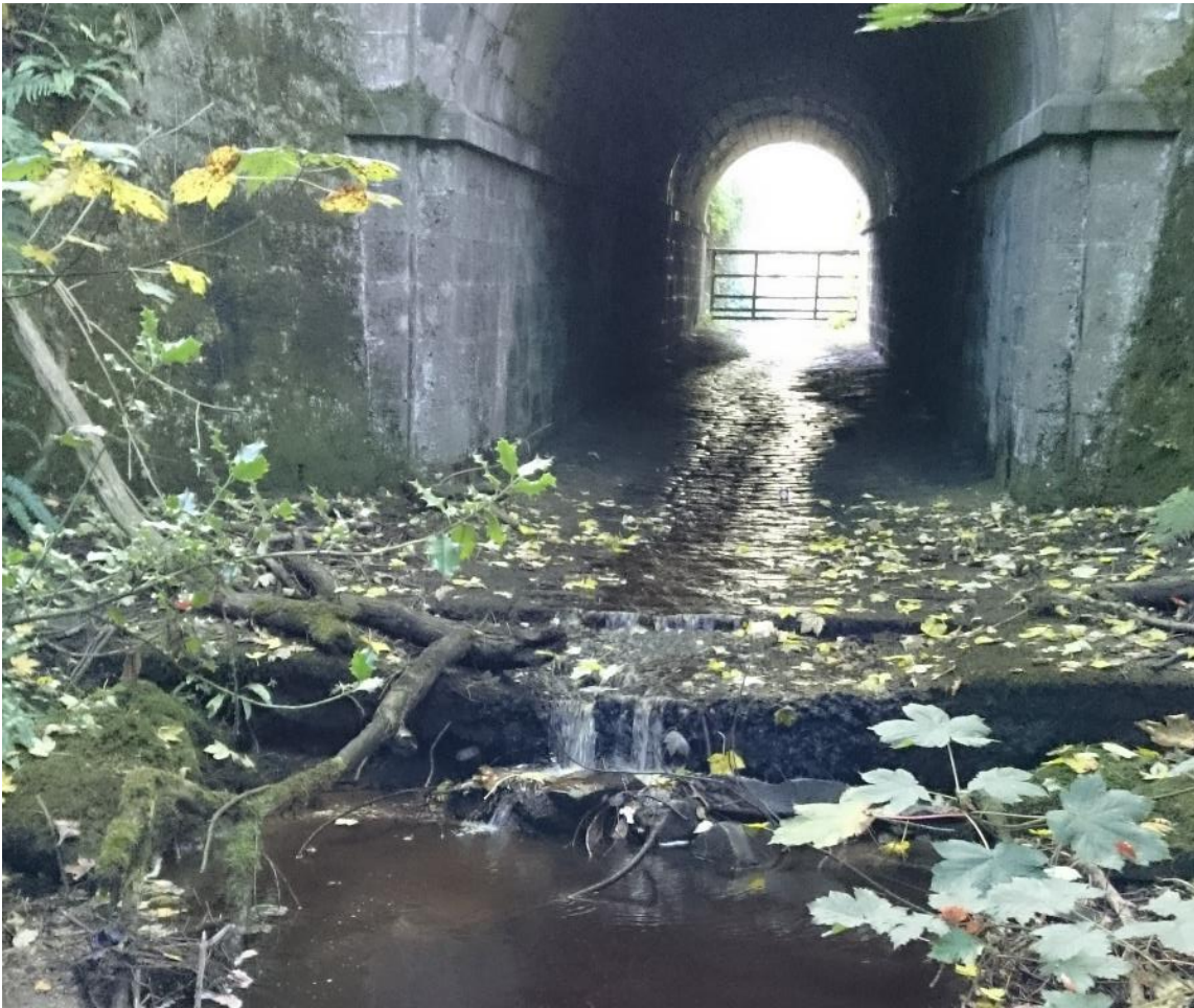
Figure 4. The stone-floored culvert under Hangingstone Rd. The head loss over the entire length of the stone-flooring (which extended approximately 25m u/s of the culvert), and including the step at the d/s side was estimated at ~5m.
