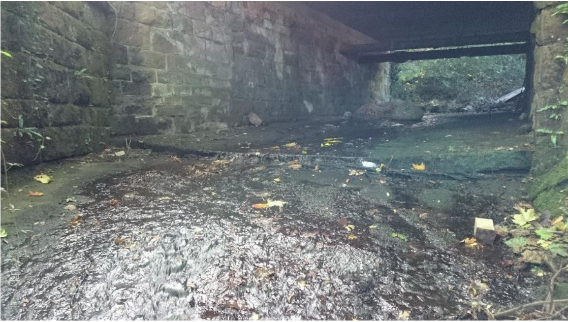
Figure 5. The concrete-floored culvert under Ben Rhydding Rd. Headloss estimated at \sim 1.8\text{m} .
