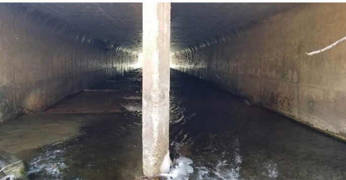
Figure 4. Condition of the Canyon Creek culvert in 2019 looking downstream. The left cell has some remaining wooden baffles originally installed in the 1970s.
