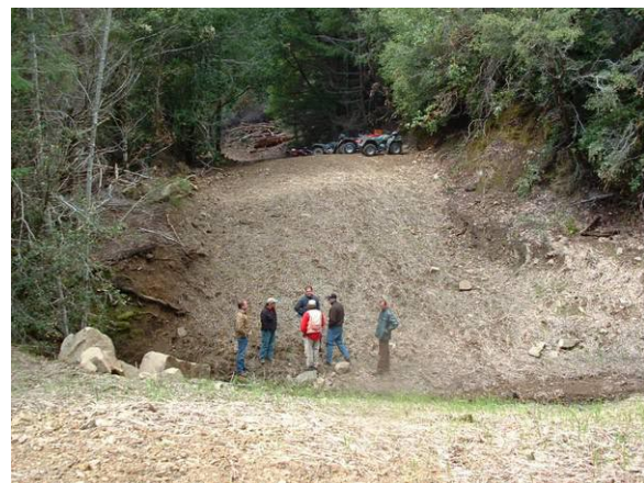
Figure 4. Decommissioned Road and Restored Stream Crossing, Hollow Tree Creek, Eel River, Mendocino County, California
