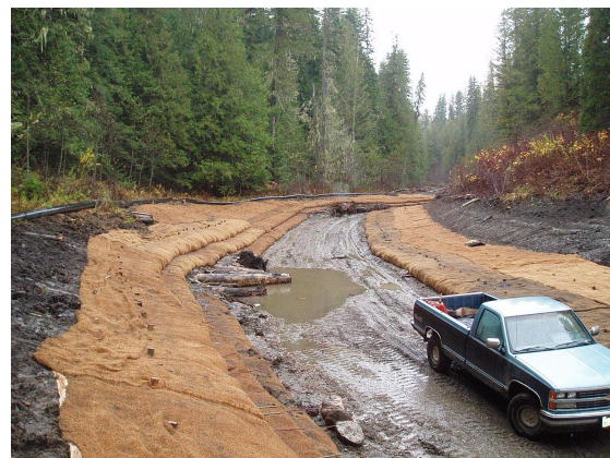
Figure 5. Fabric encapsulated soil lifts installed to stabilize stream banks (Inter-fluve, Inc. photo)
