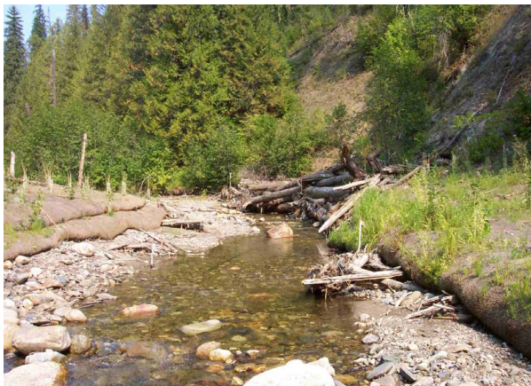
Figure 7. Channel incision occurred during a high flow event eight months following project completion
