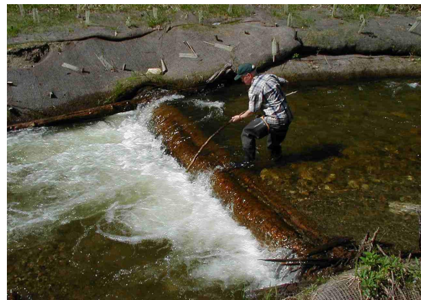
Figure 8. Significant bank erosion occurred at full span log sill, undermining the structure
