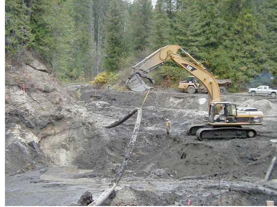
Figure 3. Flexible HDPE pipe used for dewatering was moved several times without breaking or significant leakage
