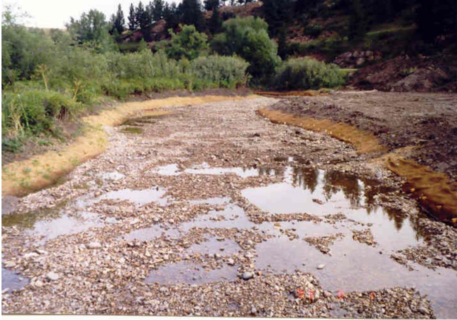
Figure 2. Prior to diversion of water into the new channel, the fabric stabilization and new gravel bottom are easy to see.
