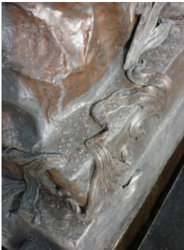
Figure 16. Detail of lead surfaces on the Neptune Fountain after applying the multilayer protective coating.
