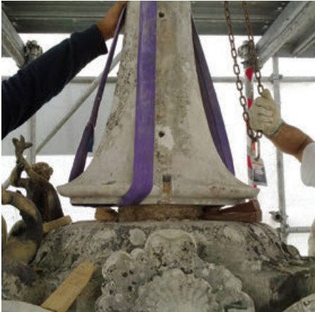
Figure 12. Removing the central block of the Medallions' Fountain to access the water distribution circuit.
