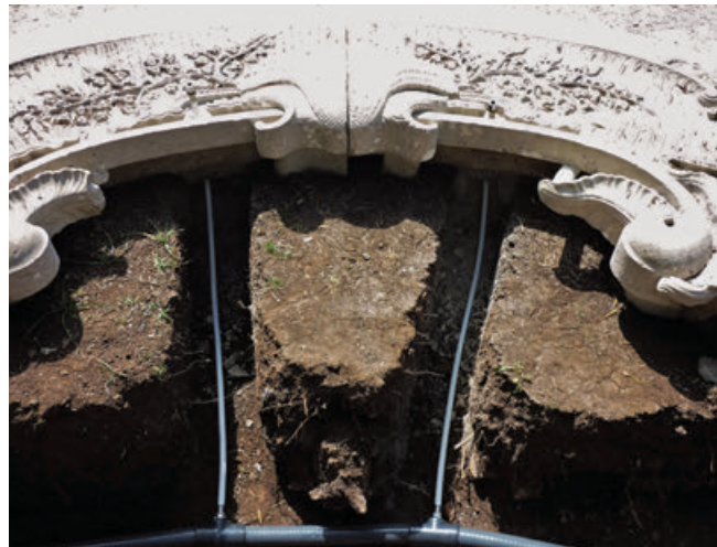
Figure 17. Replacement of the hydraulic distribution system in one of the Shell fountains.
