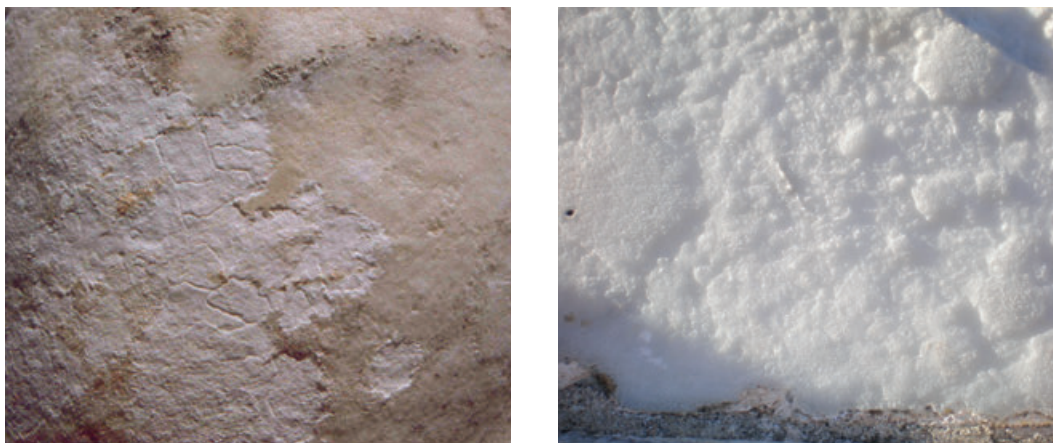
Figure 1. Surface conditions left by two different cleaning methods. Left: application of a biocide and soft brushing (area is about 30 by 40 centimeters). Right: aggressive grit blasting (area approximately 10 by 8 centimeters). Note the overall smoother surface of the stone resulting from the significant loss of original finish.
