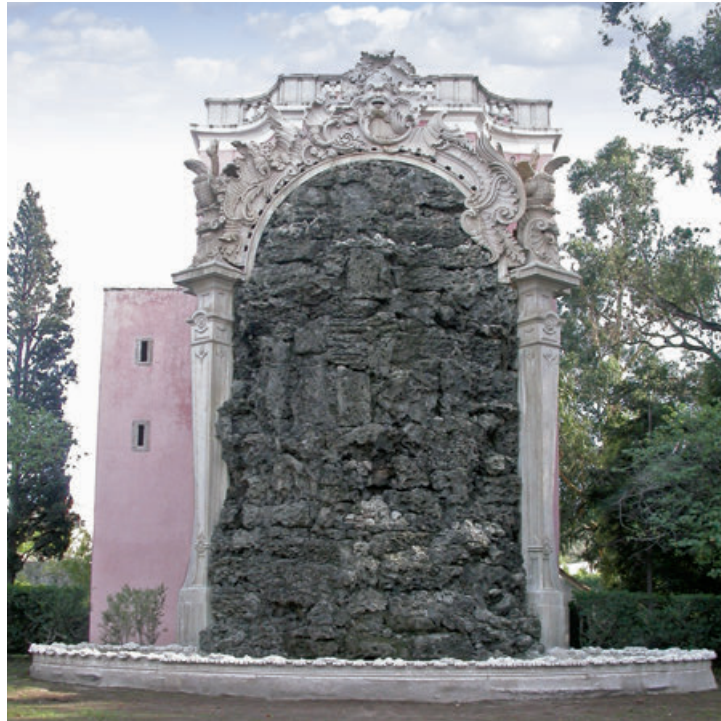
Figure 8. The Great Cascade after intervention. The water runs down the rugged stones that have been left with their acquired patina resulting from years of water circulation over them. Note that the basin has a thicker rim at its base that marks the level to which it should be buried.
