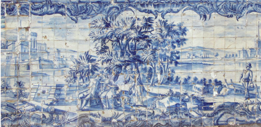
Figure 10. A closer detail of another section showing the high manufacturing quality of the tiles. The photograph also shows that many of the tiles are deteriorated and that some have been replaced, identifiable by their lesser design quality.
