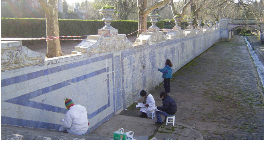
Figure 9. Condition survey of the canal. Note how close the sycamores were planted to the canal walls.
