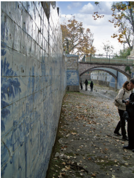
Figure 5. Rebuilt section after the 1967 flood, showing the buckling of the azulejos. The bridge over the canal corresponds to that of the center block.
