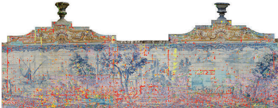
Figure 10b. Example of the condition survey of tiled canal. This survey was carried out on the maps obtained by laser scanning. Note that the major concentration of deterioration is found at the bottom of the panels, the sections that would be more frequently in touch with water during any flooding.
