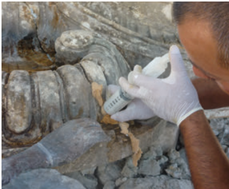
Figure 8. Grout injection into a fracture of the center “shell” of the Nereid Fountain.
