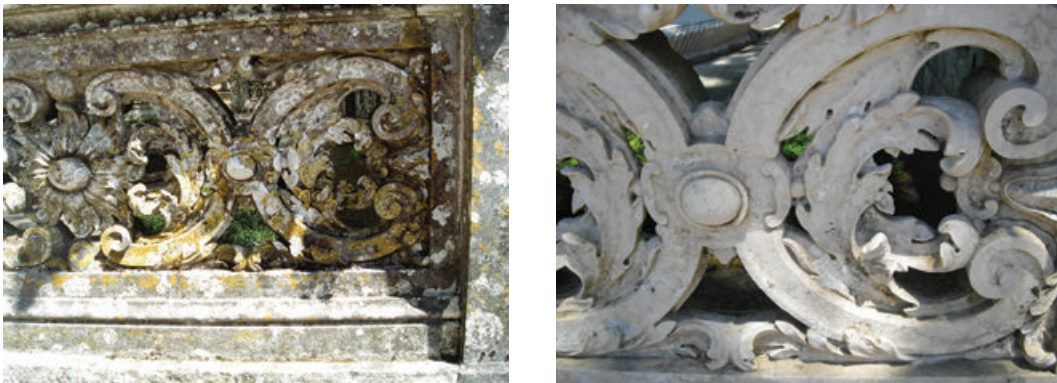
Figure 1. Balustrade of the Sycamore Plaza. Left: detail of the biological colonization prior to the application of the biocide (April 2006). Right: appearance after four years (June 2010).
