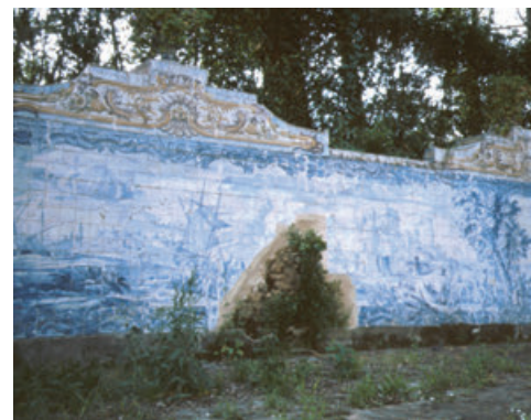
Figure 6. View of the inner west wall of the canal showing an area with azulejo loss (compare with Figure 12 in Chapter 4) partly due to the root growth of larger trees, such as poplars growing on the west bank that were propagating into the canal bed (May 2004).
