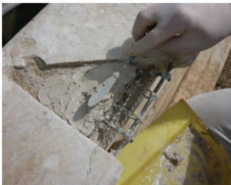
Figure 10. Filling in missing areas in the balustrade of the Neptune Fountain in the Hanging Garden.
