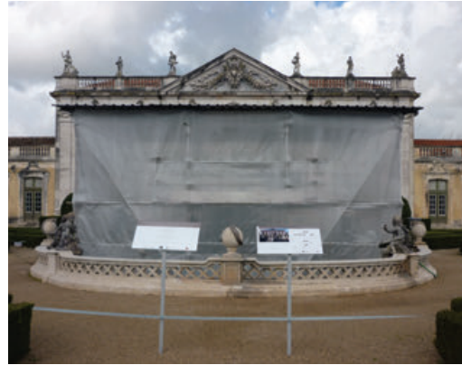
Figure 5. Scaffolding and didactic panels located at the edge of the restricted area by the Neptune Fountain.
