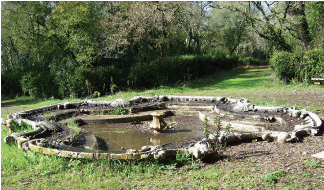
Figure 6. Condition of one of the Shell fountains prior to the conservation and restoration intervention.
