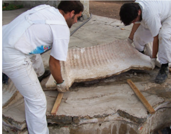
Figure 13. Resetting the decorative edge of the Dragons' Fountain by the Sycamore plaza after cleaning it, clearing out roots and debris, and leveling the base.
