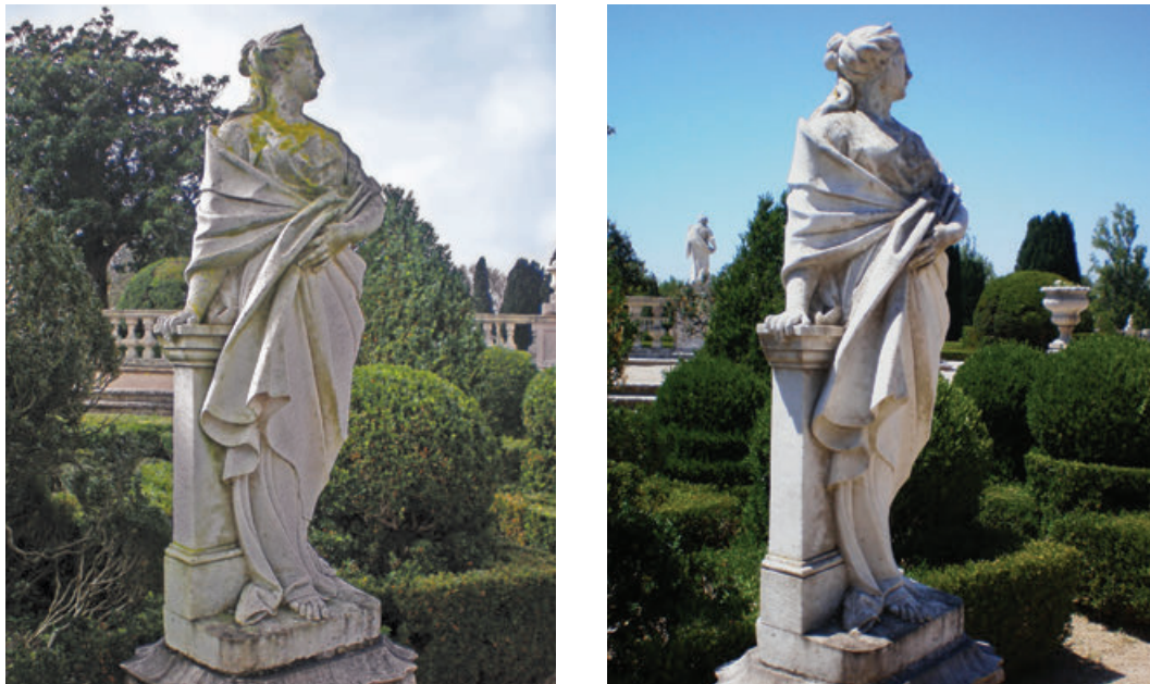
Figure 4. Architecture sculpture before a single application of Preventol 1.5% (June 2010) and two months after application. The spontaneous detachment of the colonizing lichens, particularly on head and bust has left the statue with an acceptably clean appearance.
