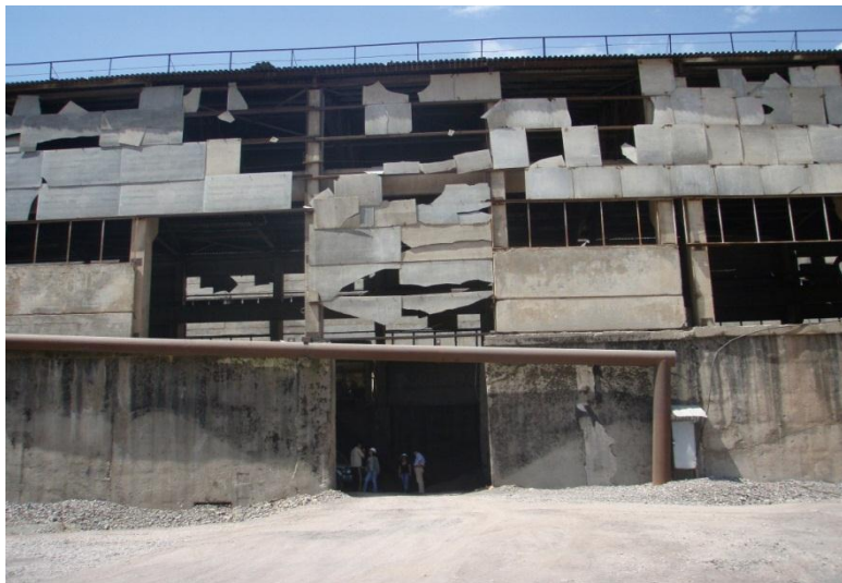
Figure 18-1: Breaker hall with largely damaged asbestos boards
