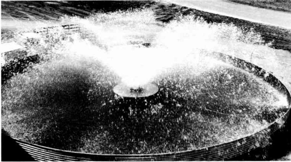
2—A cooling module is similar to an aerator except that its spray pattern is optimized for heat transfer instead of oxygen transfer. This one has a 75-hp motor, and its spray cone is about 15 feet high.
