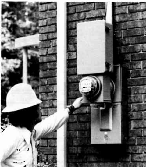
2—This prototype home transmitter/receiver for distribution-line carrier communications, shown here installed on the residence of a Carolina Power & Light Company customer, is part of the equipment used for field trials. It performs such functions as automatic meter reading, selective load control, voltage continuity monitoring, and remote service connect/disconnect.
