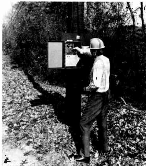
3—A prototype transmitter/receiver for use in feeder automation is also installed on the Carolina Power & Light Company system. It performs much the same functions as the home unit, but it performs them on the high-voltage part of the distribution system.
