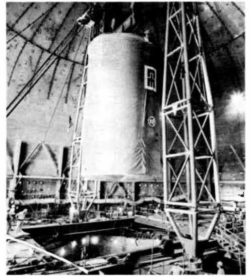
Workmen lower the Fast Flux Test Facility's guard vessel into the reactor cavity. The guard vessel is one of many safety features built into the FFTF, which will be used to test fuels and components for the nation's liquid-metal fast breeder reactors.
