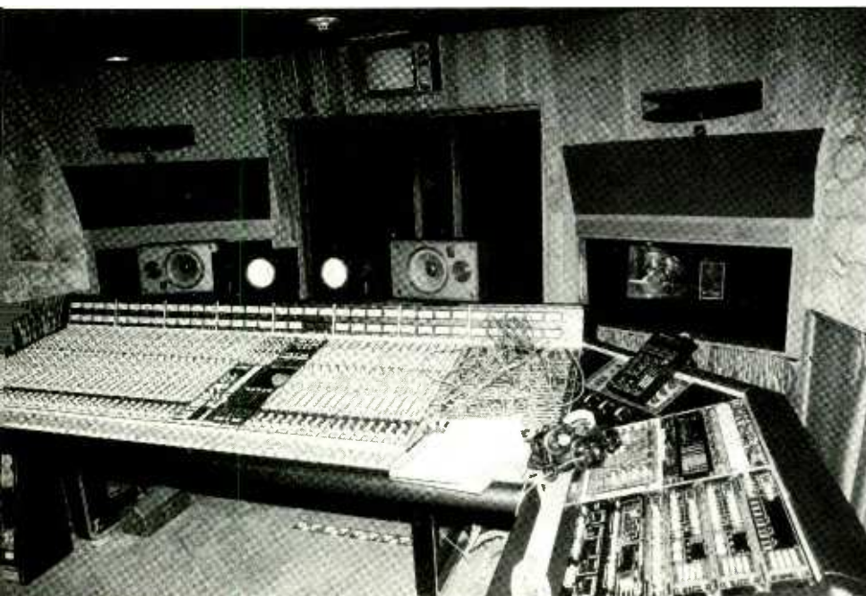
Control room after refurbishment in 1986
