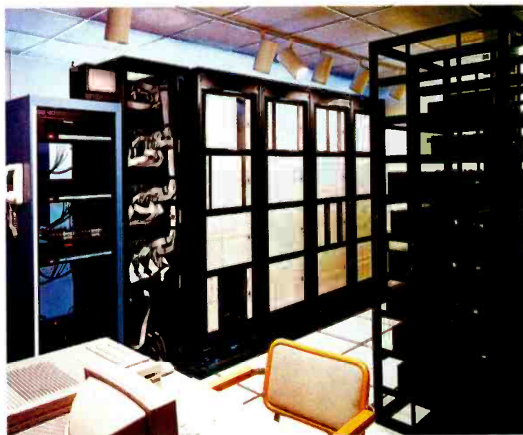
Remotely located processing racks
