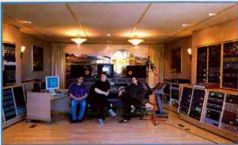
Matt Marinelli (left) of Coral Sound did wiring, system prefabrication and integration. Also pictured are acting technical director/system designer John Klett (center) and facility manager Michael Gallone.
