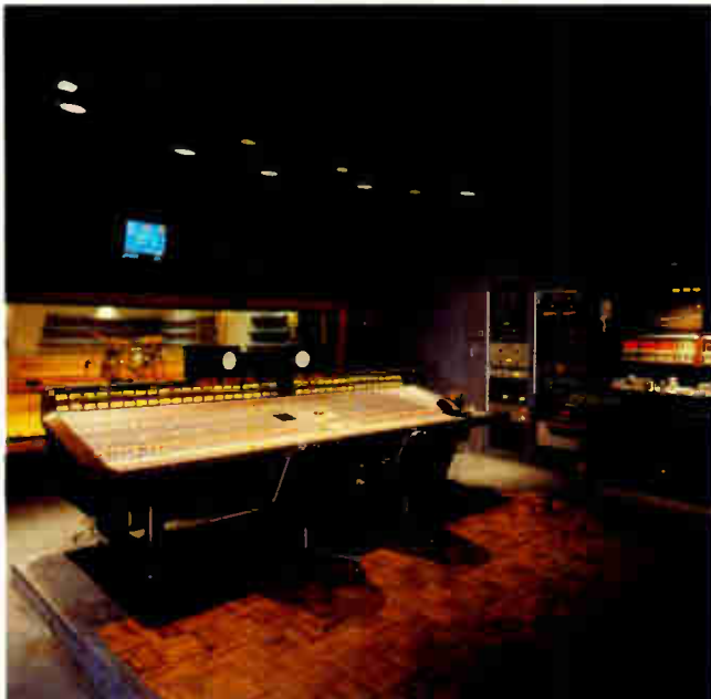
The new Studio B at Hit Factory Times Square, Manhattan, opened in September 1988. An SSL 4000G master studio system, with 56 inputs, G Series Computer and Total Recall, was added in 1989.
