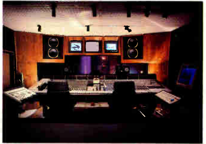
Manhattan Center Studios' Studio 7 in New York City now features an SSL G Series/56 and Richard Rose-designed monitoring systems with soffited, shock-mounted Tannoy FSM-U mains and Tannoy AVM near-fields.
