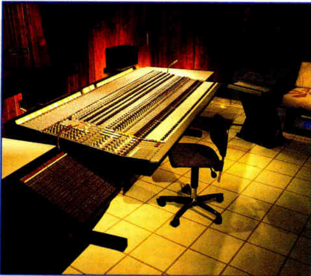
CONTROL ROOM I
