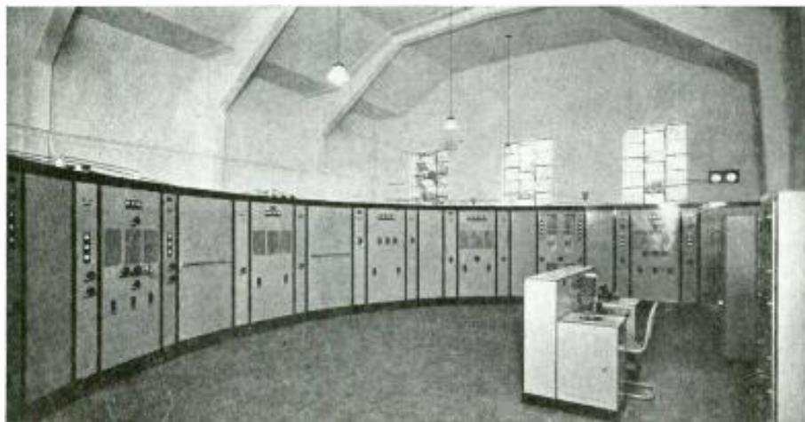
Interior view of the transmitting station of PRA8, Radio Clube de Pernambuco, Brazil, showing the short-wave control panels and supervisor's desk.
