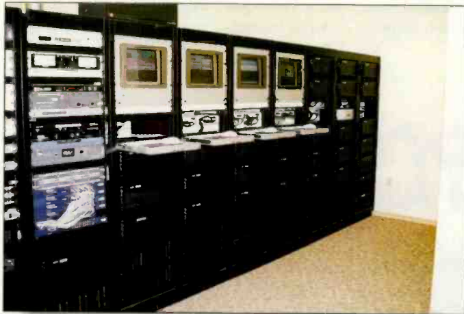
By locating the servers in a common space, the noise and heat are contained, and service and maintenance are simplified.
