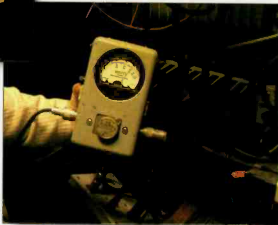
When the work is finished, verify the power levels for both forward and reflected power.
