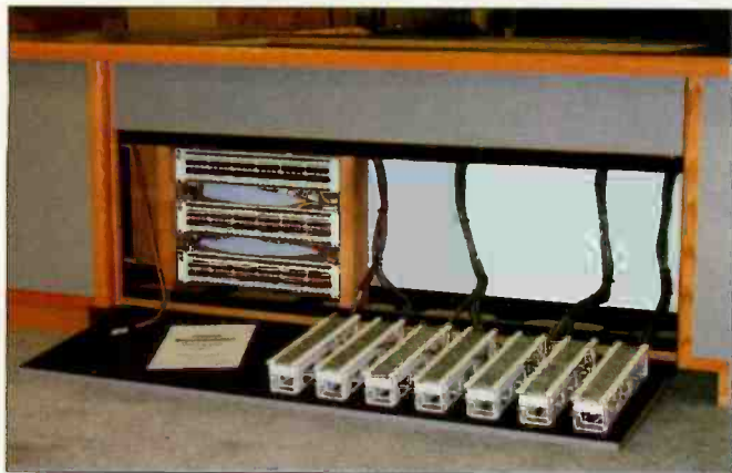
Studio furniture must not only support the equipment installed in it but also serve as a cable raceway and termination point.
