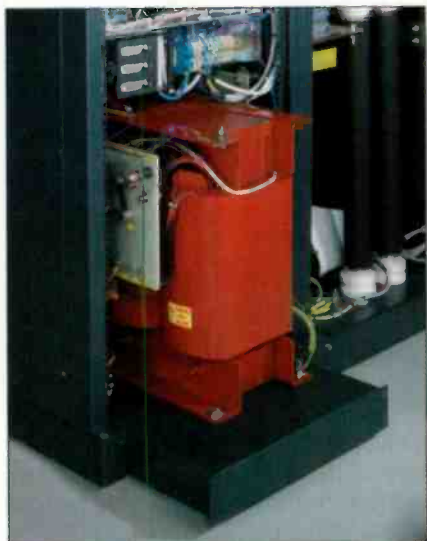
The high-voltage power supply rolls out for easy access.
