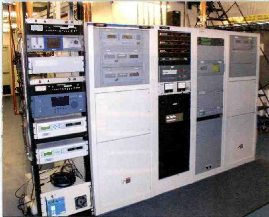
The transmission equipment was also part of the facility upgrade. New transmitters were installed to transmit analog and HD Radio signals.
