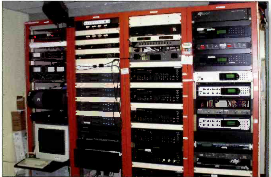
The Network Area features recording and terminal equipment for WLRN's radio and TV operations. Satellite IRDs receive and demodulate NPR feeds for immediate on-air playback, while various Sony and Tascam devices record other programs to air at a later time.
