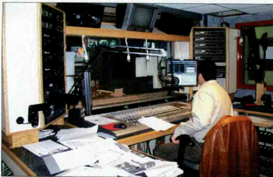
The radio portion of WLRN's master control center features a Harris PR&E B-MX digital with analog and digital outputs, allowing the station to broadcast in HD Radio and analog FM.
