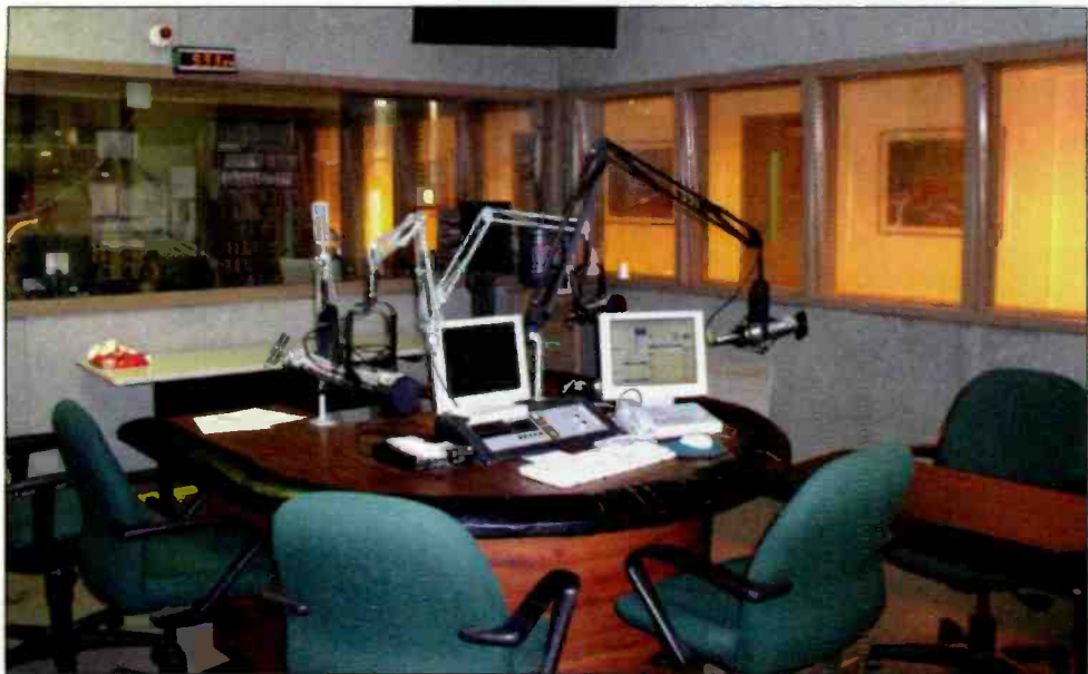
In lieu of traditional routing systems, sources from the talk studio — which often originates live programming — are hard-wired to the master control console.
