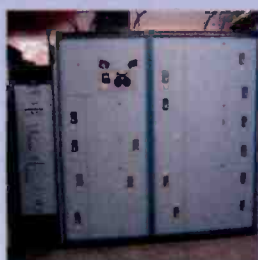
Kintronic Phasor Cabinet/ Control Rack Installed At KNWC-AM 5/2.3kW 1270kHz Five Tower DA-2
