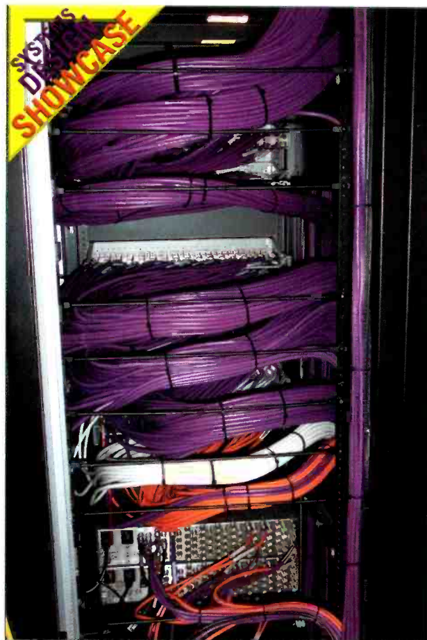
A rack in the technical core area shows well-planned wiring paths, and wires color coded for varying signal types. Where practical, wiring is nested into the 4-inch space between racks, to improve access to equipment rear panels.
