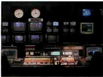
KJLA Los Angeles, California Ross Synergy 3, RossGear Terminal Equipment
