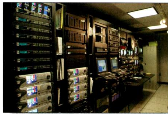
Video levels are checked via a Videotek VTM-150 on multiple LCD monitors. Audio monitoring is provided by Wohler AMP2-AM/AMP2A-4S audio meters and a PTV PT0600C-11 stereo correlation meter.
