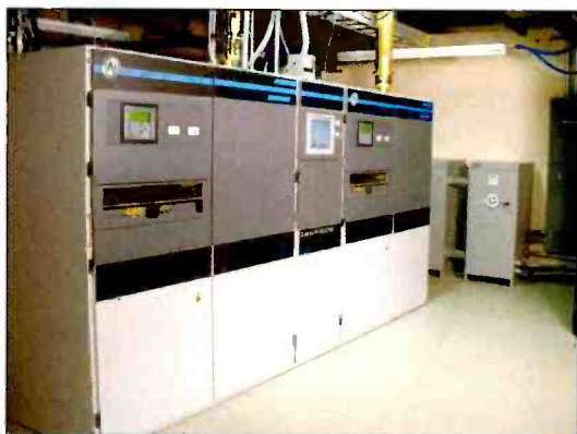
When WTTA-TV in Tampa, FL, installed an Ai two-tube ESCIOT depressed collector analog/digital transmitter last June, it saved $13,000 per month in operating costs.
