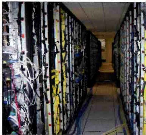
The new media server and patch panel provide the facility with 300 hours of news video with redundant backup.
