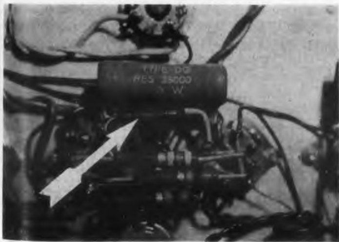
Fig. 2: Precision resistor placed adjacent to a power dissipating unit will exceed temperature coefficient rating.
