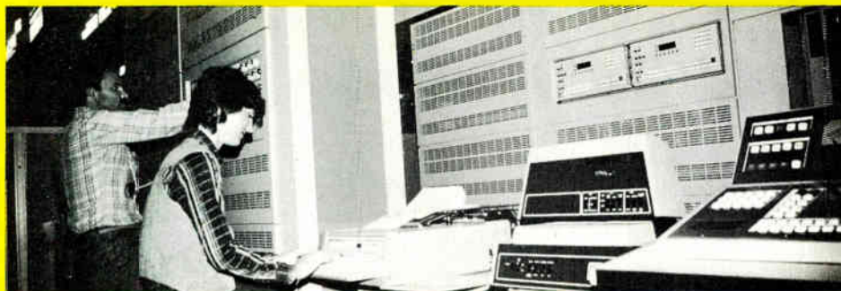
NEAX 61 ESS in service at the Manteca Central Office of Continental Telephone of California
