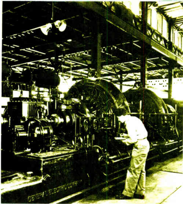
Sources. Alexanderson alternators at RCA's Rocky Point, N. Y., transmitter once carried the whole load of overseas radio traffic.
