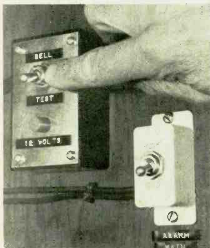
This simple and effective test unit consists of a small box containing a DPDT toggle switch, part of the original equipment, is for the alarm bell. The white switch part of the original equipment, is used to arm and disarm the detection system from inside the house. Use lamp cord or 12-volt bell wire to connect these units.
