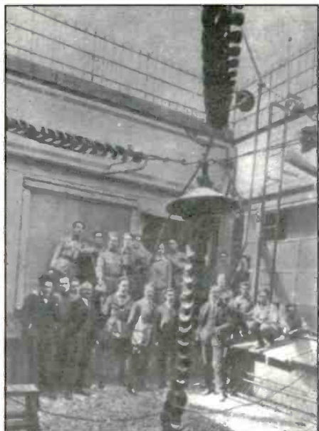
Station FL's personnel near the huge lead-in wire and insulators at the tower's base.
