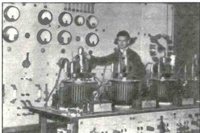
The mercury turbines for manipulating arc at the original FL. Behind is the control switchboard of the arc transmitter.
