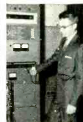
John Radtke, Sherwood's Chief Research Engineer, checks out WKFM's stereo multiplex transmitting equipment.
