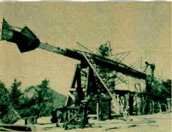
1. KNXT ANTENNA IN PROCESS OF PREPARATION for erection atop its 160-foot tower. Tower itself was anchored fourteen feet into the ground in nine-by-nine holes. Total height, 243 feet. These pictures taken by Bob Bullock, one of transmitter engineers.
