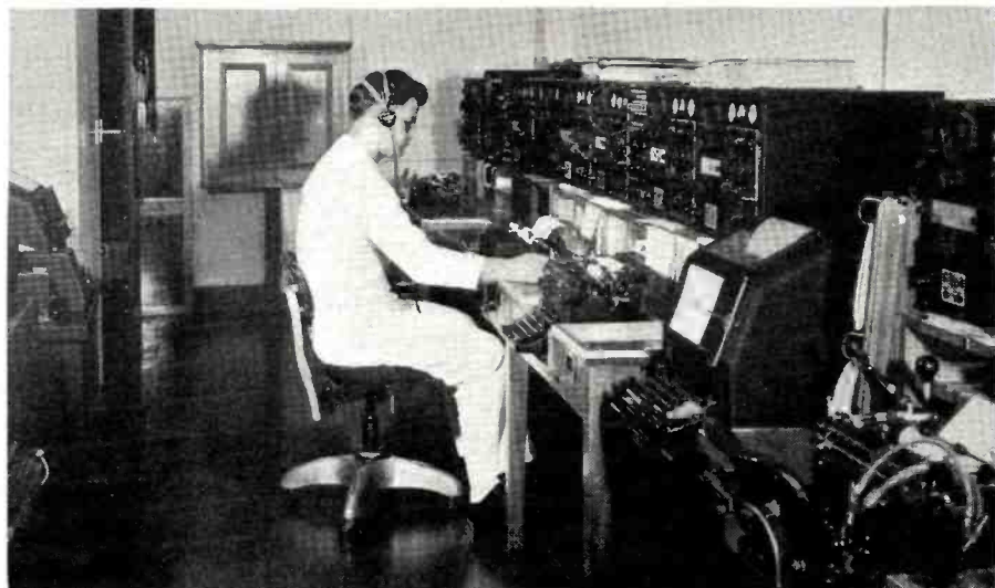
Fig. 2. A naval communication room at the Cheltenham, Maryland, Naval Radio Station. In this installation both manual equipment and the newer radioteletype units are used.
