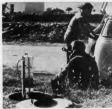
European engineers of the International Telephone and Telegraph Corporation work on installation of a buried transistor repeater for a carrier telephone system in Sardinia using a new type of coaxial cable that is thinner than a pencil.
